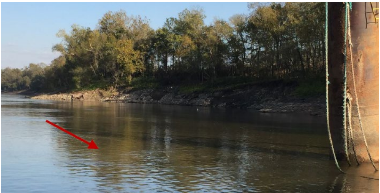
Figure 4: Bank failure adjacent to a structure
