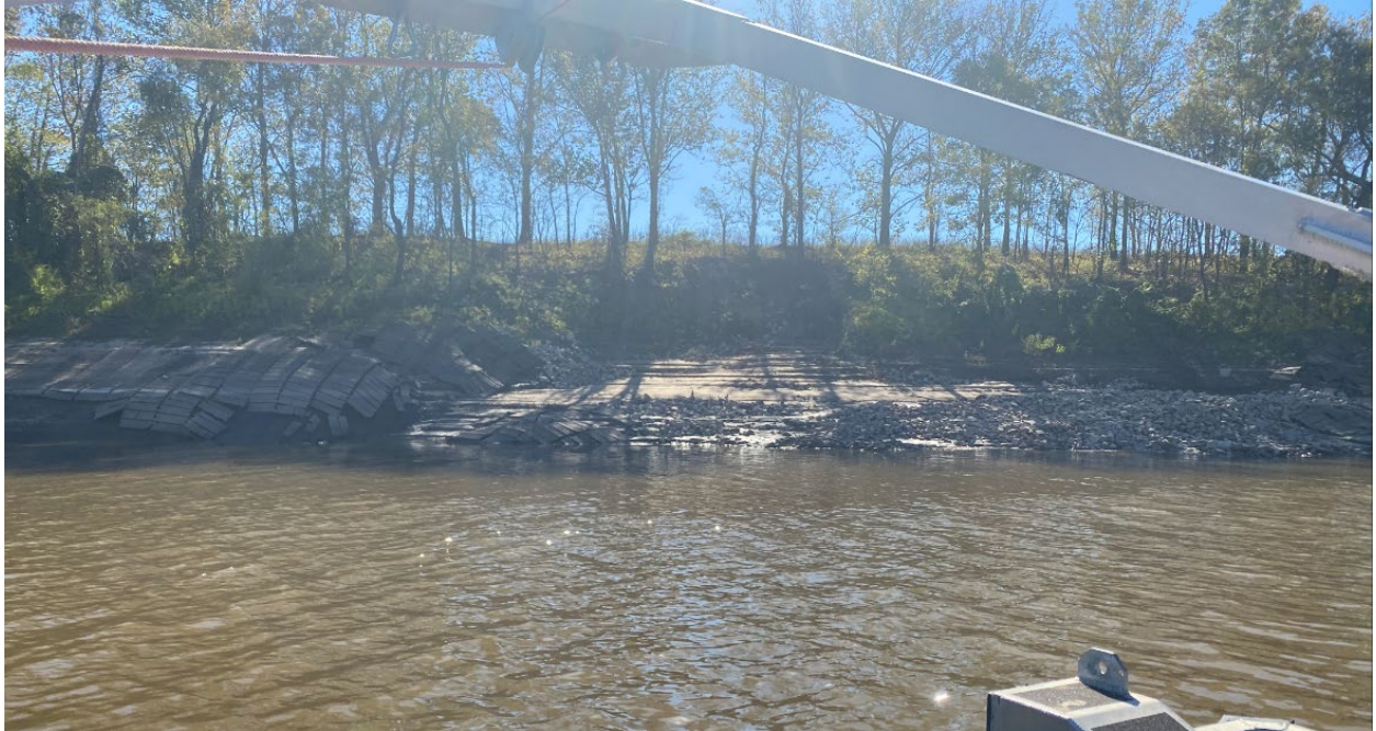
Figure 1: Failed revetment along the Red River
