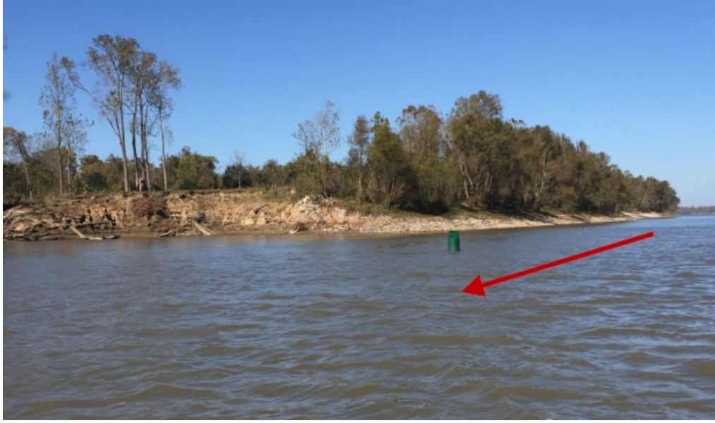
Figure 3: Bank failure adjacent to revetment
