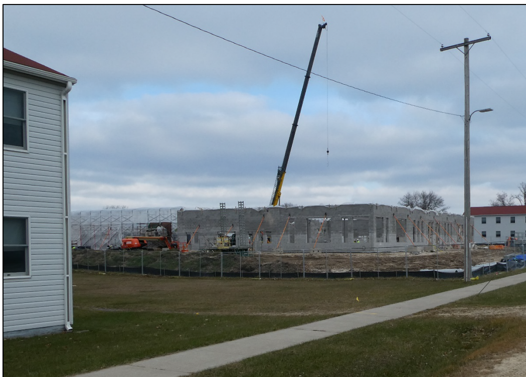
Figure 30. Looking north at a not-yet-numbered mess hall under construction between the 2400 and 2500 areas between West 12th and West 13th Avenues, 2020 (ERDC-CERL 2020).
