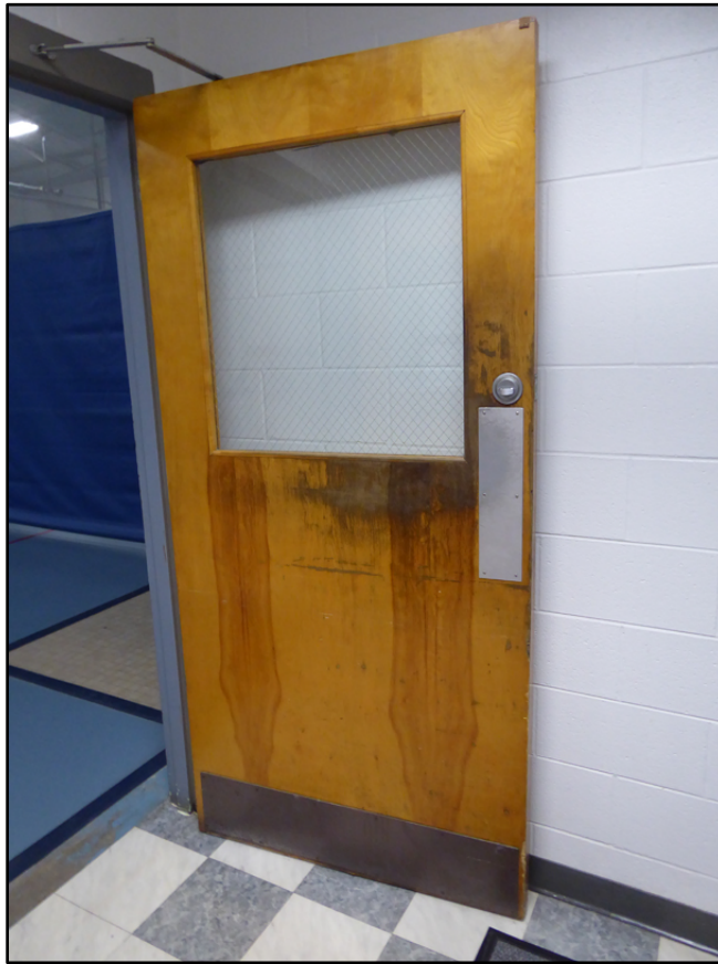
Figure 43. Typical original blonde-wood interior door with a large pane in the top half of the door in Building 1122, Rumpel Fitness Center (ERDC-CERL 2021).
