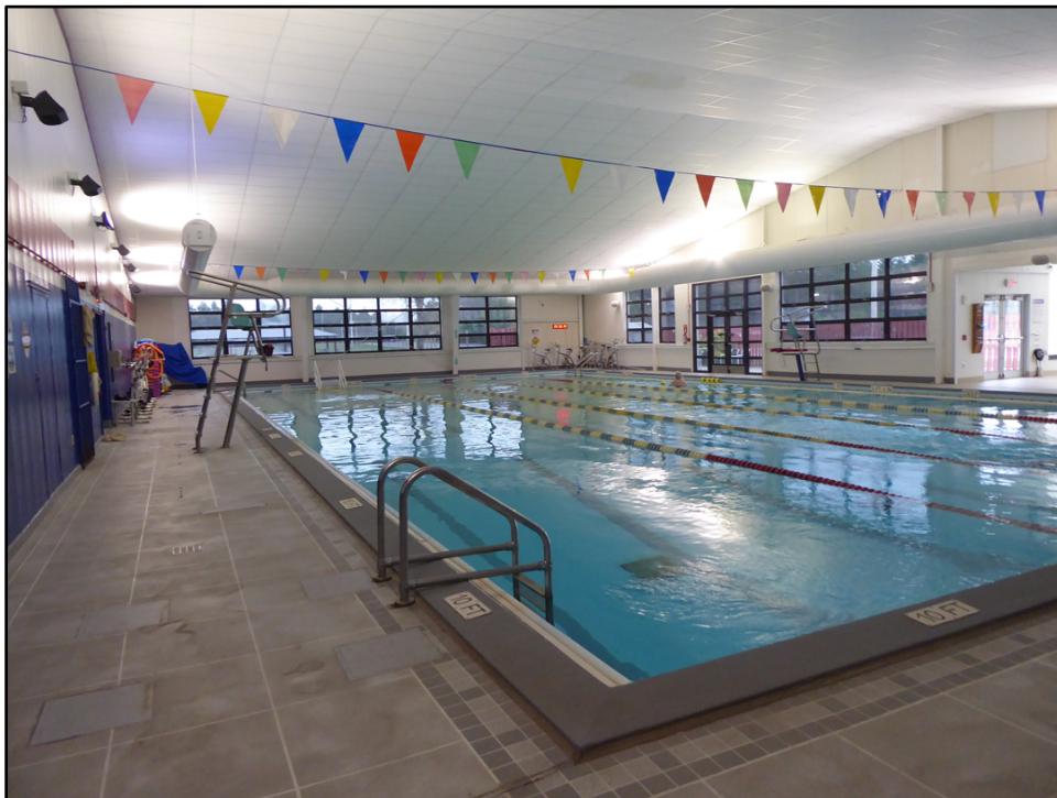
Figure 40. Interior view of the pool area in Building 1122, Rumpel Fitness Center (ERDC-CERL 2021).
