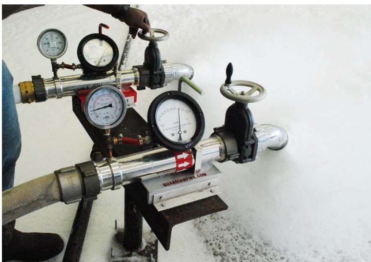
Figure 3. Guardian Flowmeter Stands Discharging Foam
