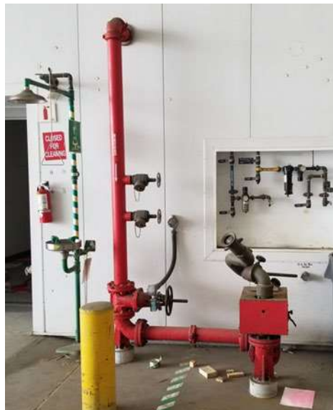
Figure 2. Hangar Bay Fire Suppression Floor Monitor and Valves
