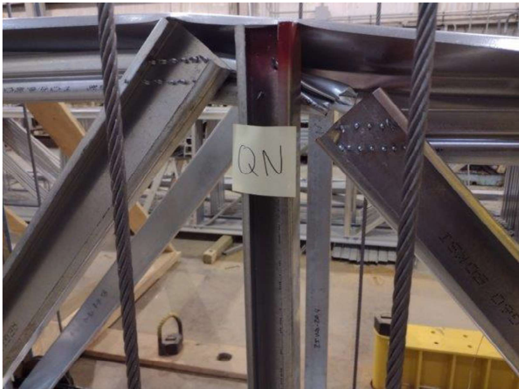
Figure 40: Beginning of Tension Chord Separation (AG48-D57)
