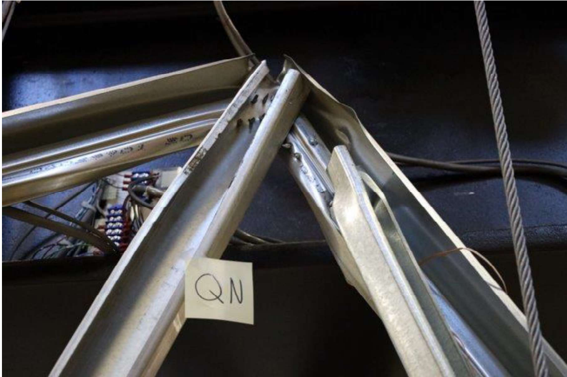
Figure 34: Partial Tearing in Tension Chord at Joint QN (AG48-D35)
