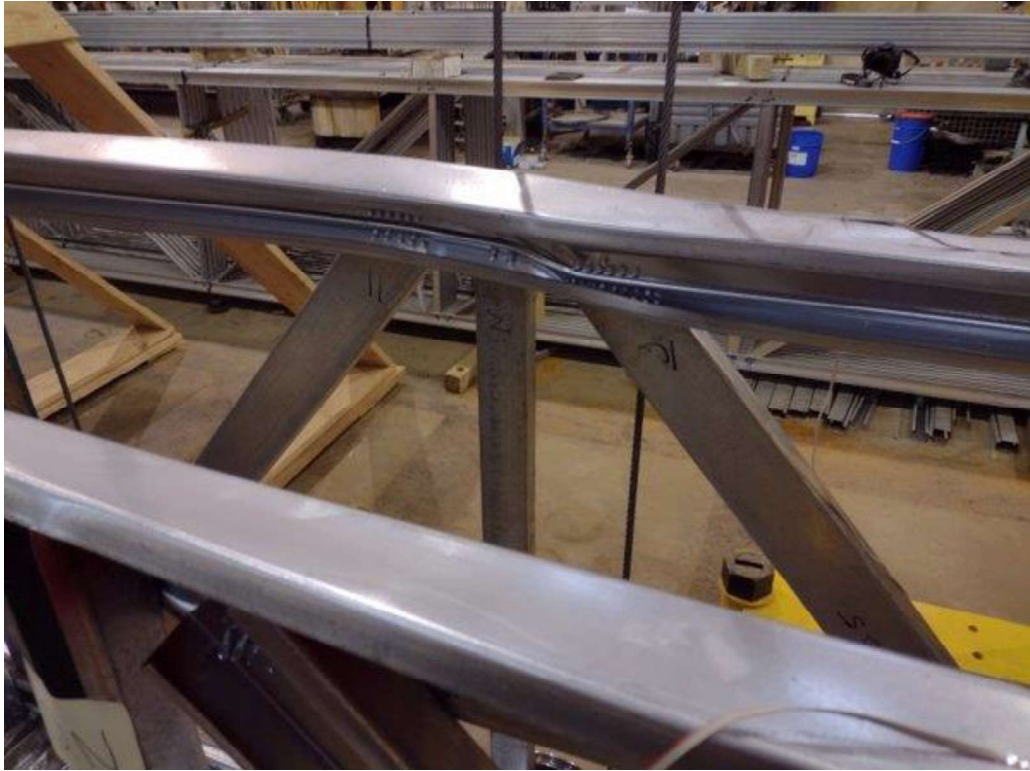
Figure 39: Initial Tension Chord Deformation (AG48-D57)
