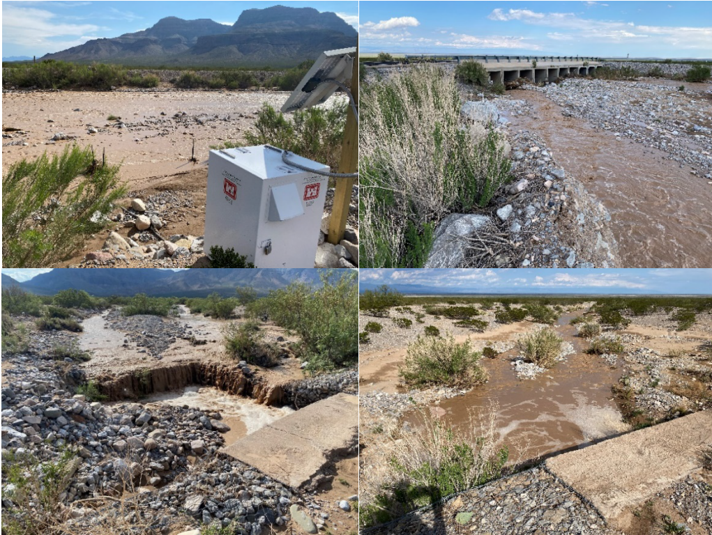
Figure 18. 7 July 2021 flood event at downstream gauge station ( top left ), upstream face of culvert 1 ( top right ), culvert 2 looking upstream ( bottom left ), and culvert 2 looking downstream ( bottom right ).
