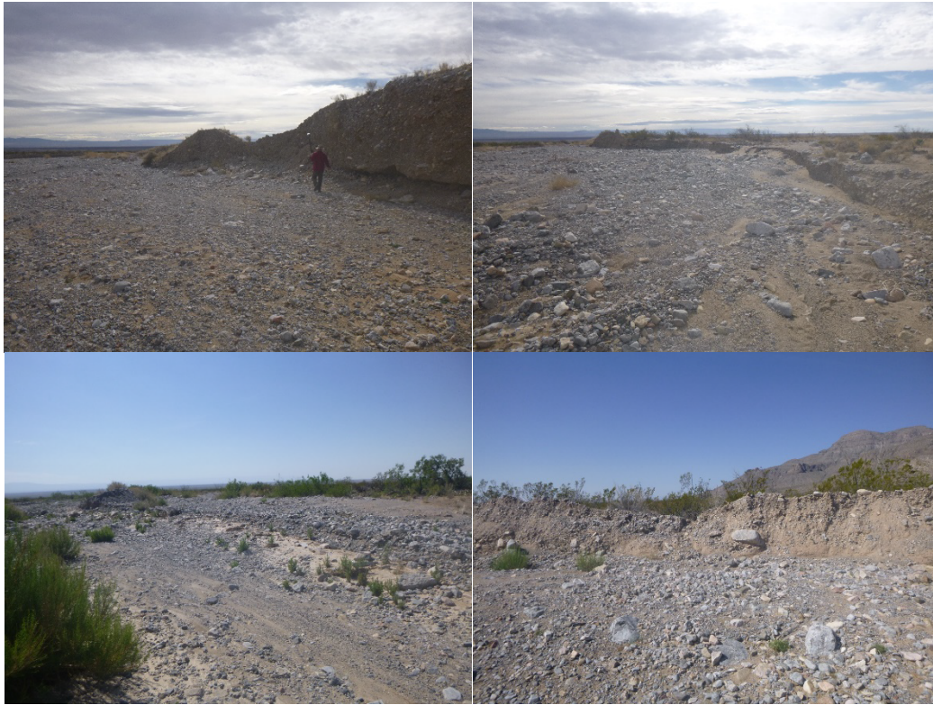
Figure 34. Scour locations 1–4 (starting top left , clockwise) as of March 2022.
