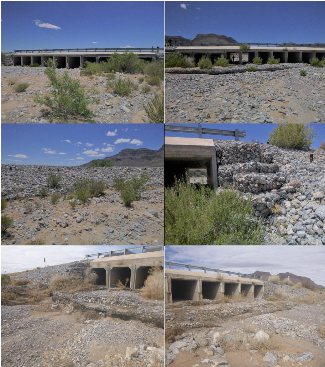
Figure 4. Culvert 1 upstream and downstream faces ( top left and top right , respectively). Reinforced section of main berm ( middle left ) and gabion baskets ( middle right ). Gabion mattress scour BMP and toe scour ( bottom ).
