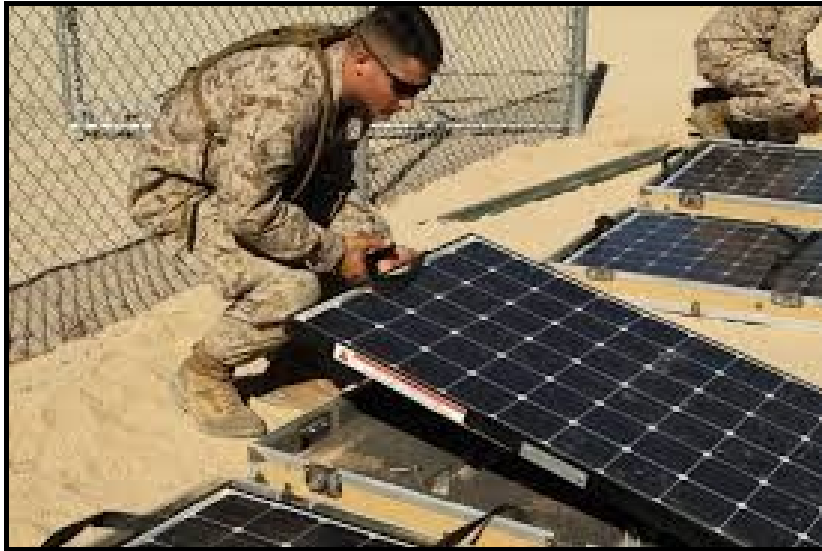
Figure 30: Solar Portable Alternate Communications Energy System (SPACES).
