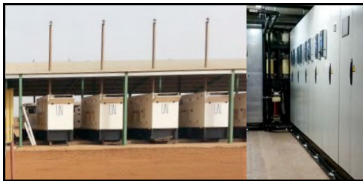
Figure 6: Deployable Power Module.
