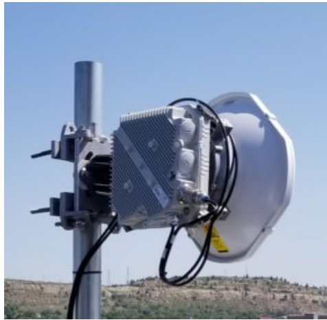
Figure 21. The BridgeWaveFlex4G-1000 used for point-to-point communications.
