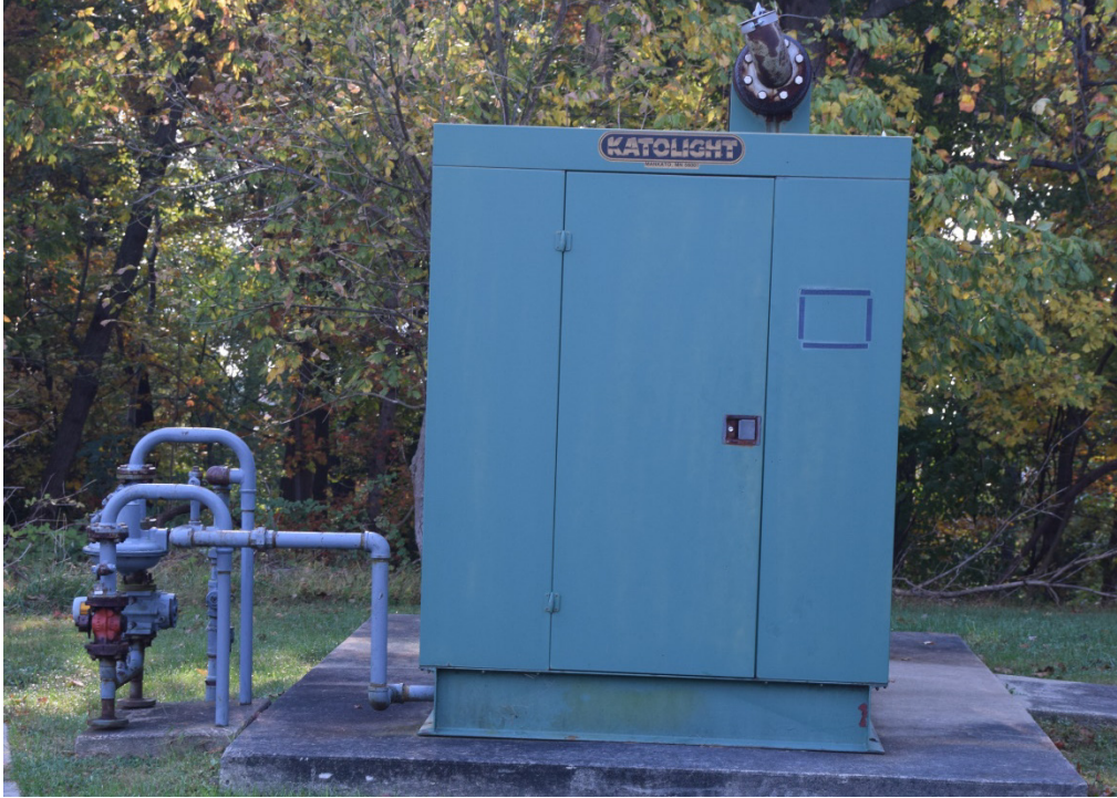
Figure 5. Existing Building E Generator
