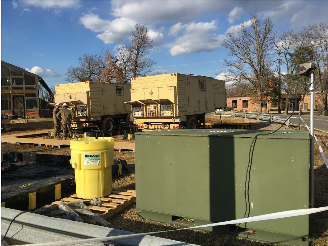
Figure 11. Location of Mobile Temporary Generation (L) and 2.0 MVA Transformer (R) Adjacent to Building L
