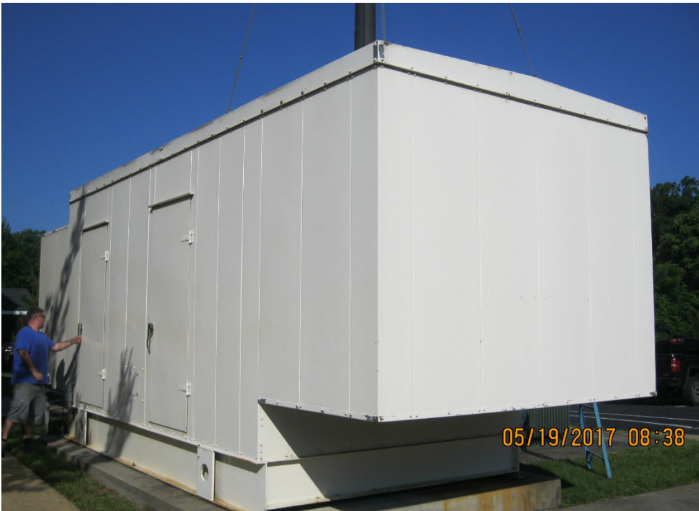
Figure 6. Existing Building I Generator (375kW)
