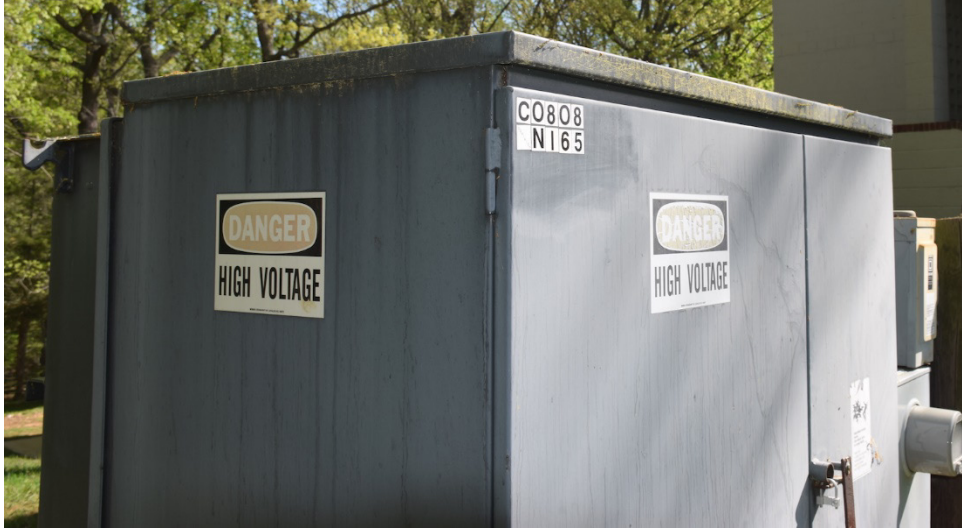
Figure 3. Existing Transformer at Building A
