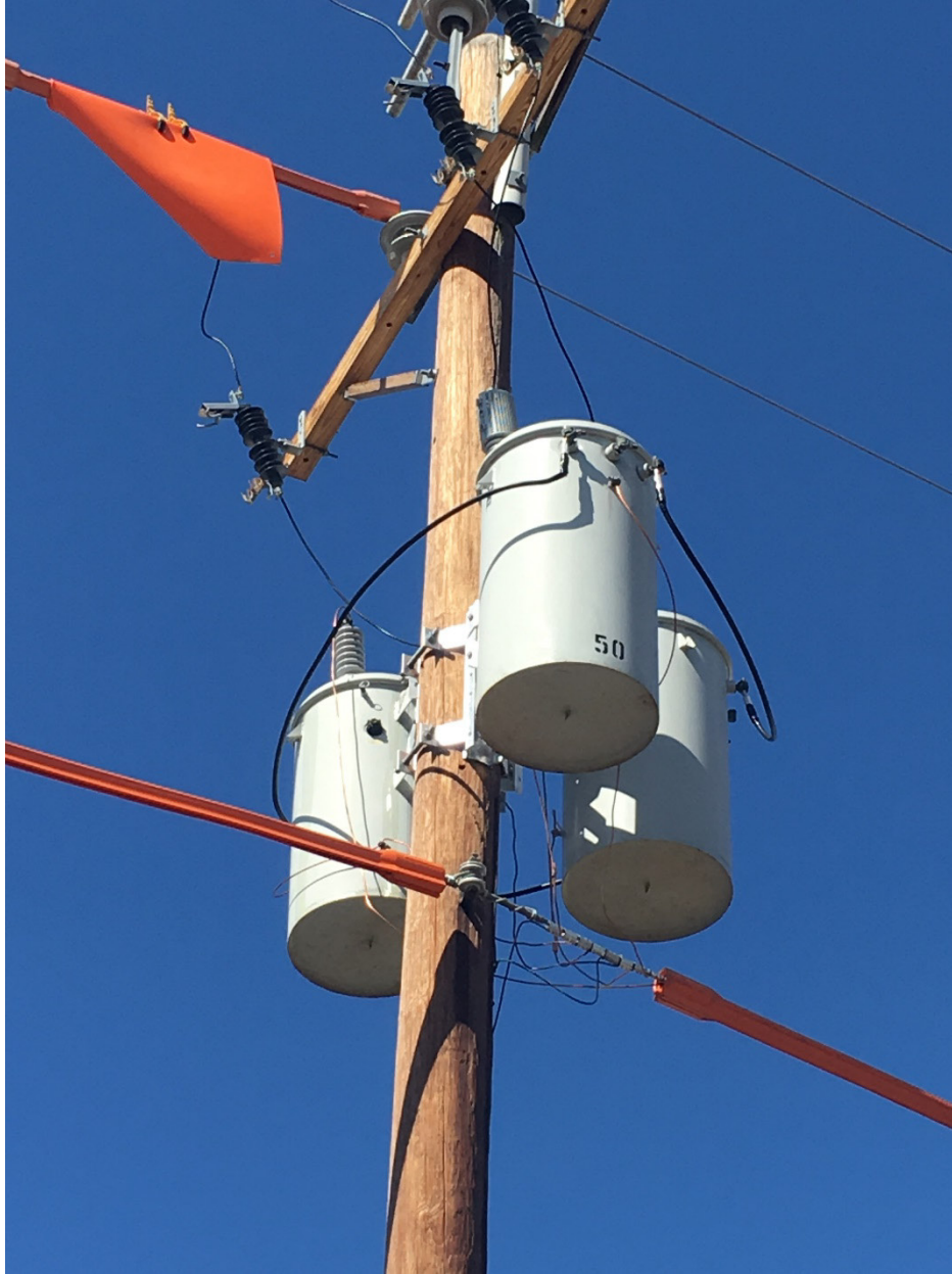
Figure 10. Pole Mounted Grounding Transformer near Recloser R3
