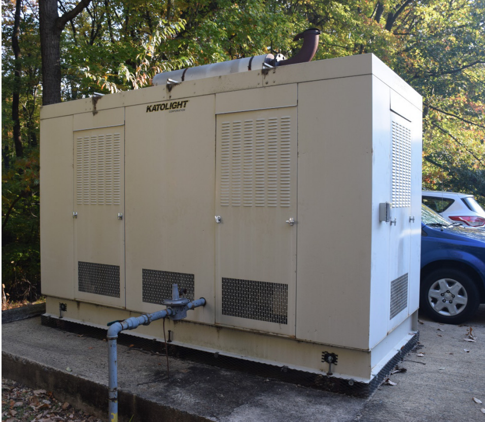
Figure 4. Existing Building A Generator (325kW)
