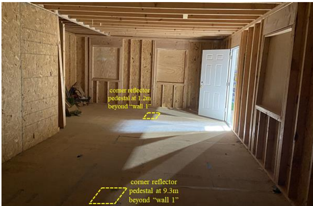
Fig. 10 Inside the plywood building: locations of corner reflectors toward/away from antenna pair T_{X1}/R_{X1}
