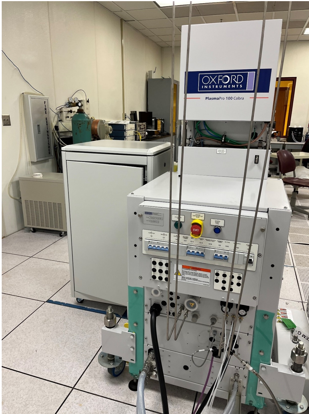
Figure 2. The backside of the installed PlasmaPro 100 Cobra ICP etching system which are connected with power, water, compressed air, process gas, nitrogen gas, helium gas, chiller, and vacuum.
