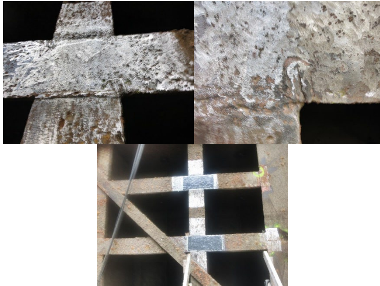
Figure 15. Crack pattern and CFRP repairs at locations 3 and 4.
