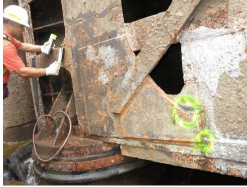
Figure 3. Poor welding quality at diagonal gusset plate (river side).
