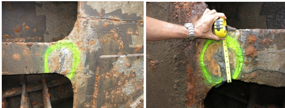
Figure 4. Crack at end diaphragm downstream flange with tapered end section flange and at end diaphragm downstream flange with girder flange.
