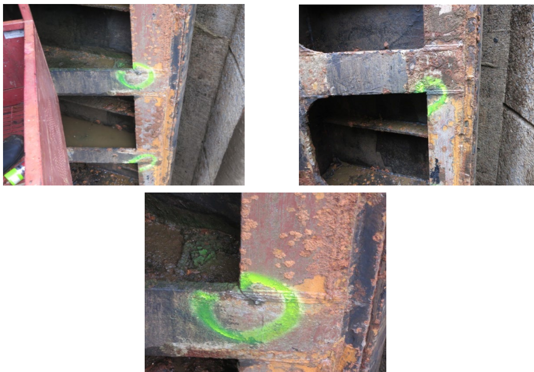
Figure 6. Cracks at downstream tapered end section flange and end plate flange.
