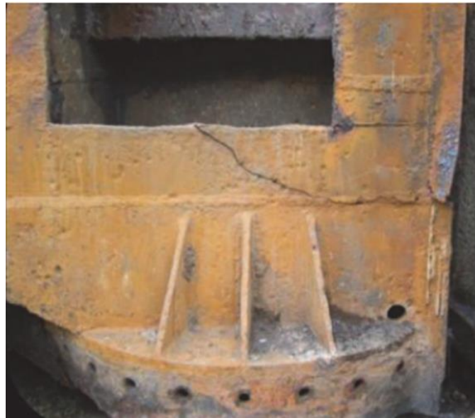
Figure 1. Crack near the pintle socket of a miter gate (Mahmoud and Riveros 2013).
