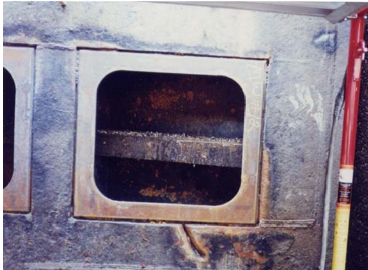
Figure 3. Welded window frame-type repair implemented for gates at the Markland Locks and Dam.
