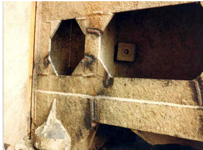
Figure 2. Cracks repaired by rewelding in miter gate girder and diaphragm flanges that experience compression loads during gate operation (USACE 2010).
