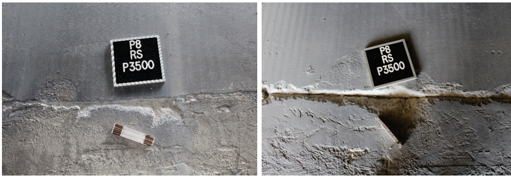
(a) Joint spall at north edge
