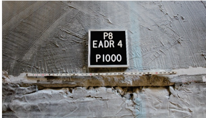
(a) Joint spalling at 1,000 passes
