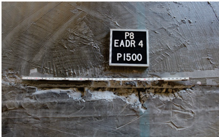
(b) Joint spalling at 1,500 passes
