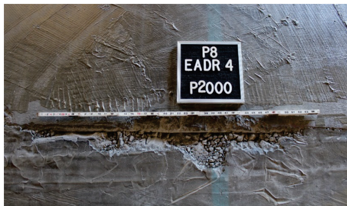
(c) Joint spalling at 2,000 passes
