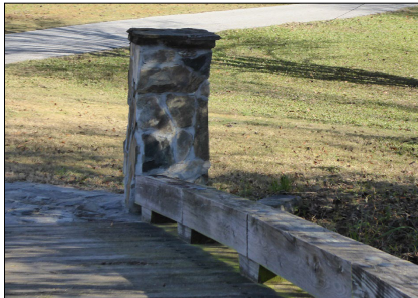
Figure 65. View of LAKE7, which is a glue lam and timber decked bridge erected in 2009. (ERDC-CERL, 2020. Public domain.)
