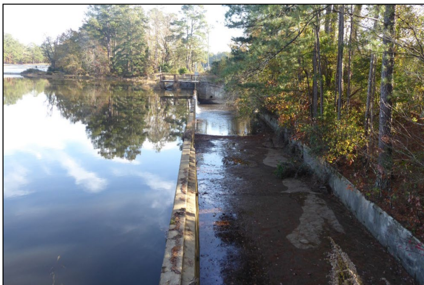
Figure 46. Looking north along the spillway on Gordon Lake Dam. (ERDC-CERL, 2020. Public domain.)
