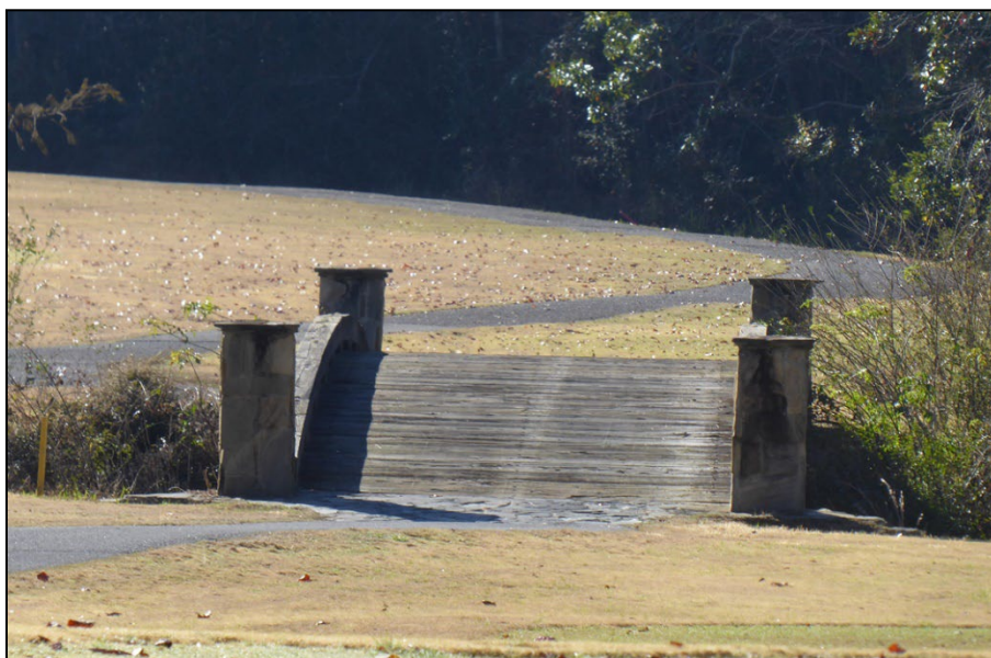
Figure 64. View of LAKE3, which is a glue lam and timber decked bridge erected in 2009. (ERDC-CERL, 2020. Public domain.)
