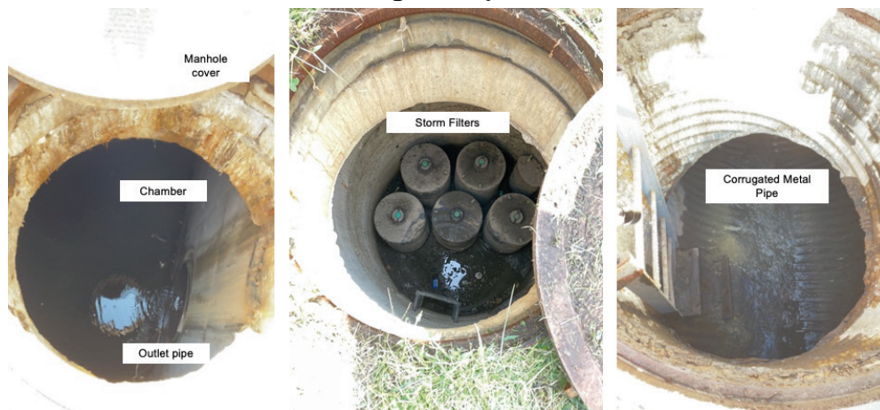
Figure 1. Example of the US Army Garrison (USAG) West Point chamber and filter underground systems.
