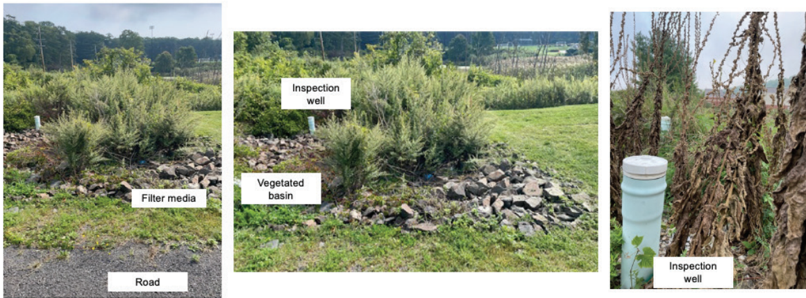
Figure 2. Example of sand filter components at USAG West Point.
