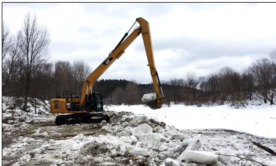
Figure 32. Example of long boom excavator removing jammed ice, weakening the toe of an intact jam in Johnson, Vermont (Photo: Eric Osgood, used with permission).
