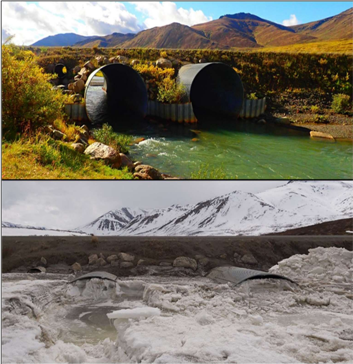
Figure 41. Culvert icing in oversized culverts. (Image reproduced with permission from Burrell et al. 2021.)
