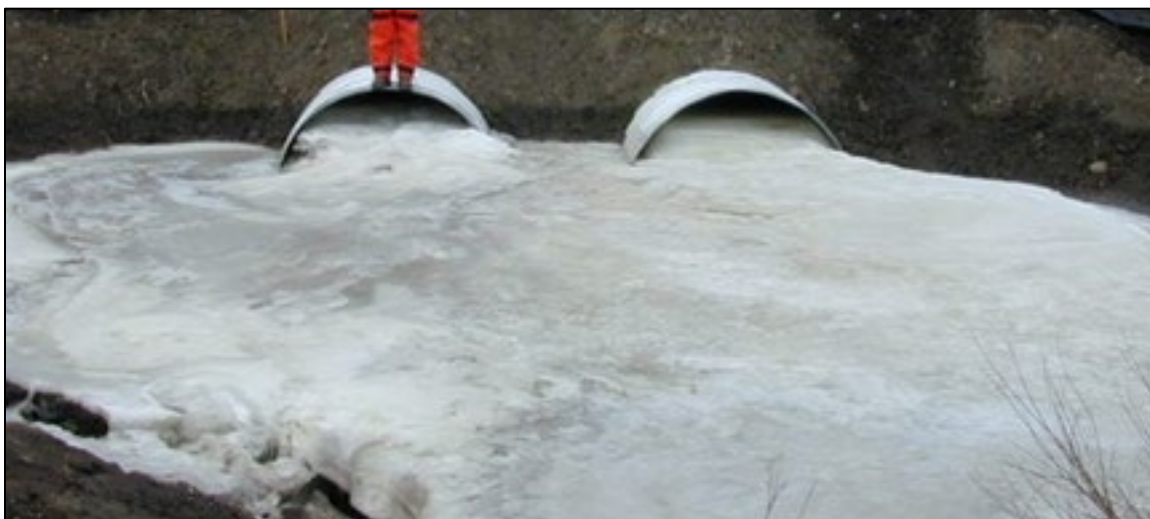
Figure 6. Road culverts obstructed by aufeis, Alberta, Canada. (Image reproduced with permission from F. Hicks.)
