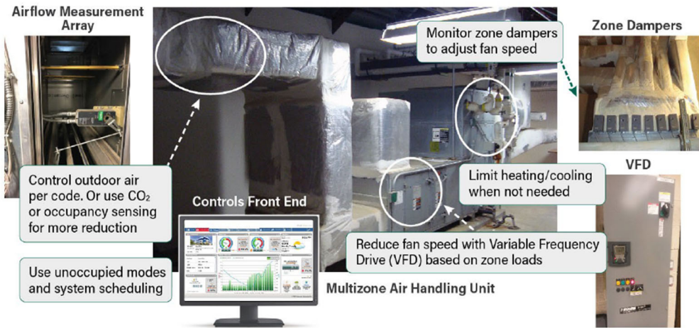
Highlights of Control Changes to Multizone Air Handler
