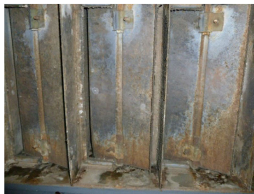
Rusty damper blades still work in 40-year-old unit.
