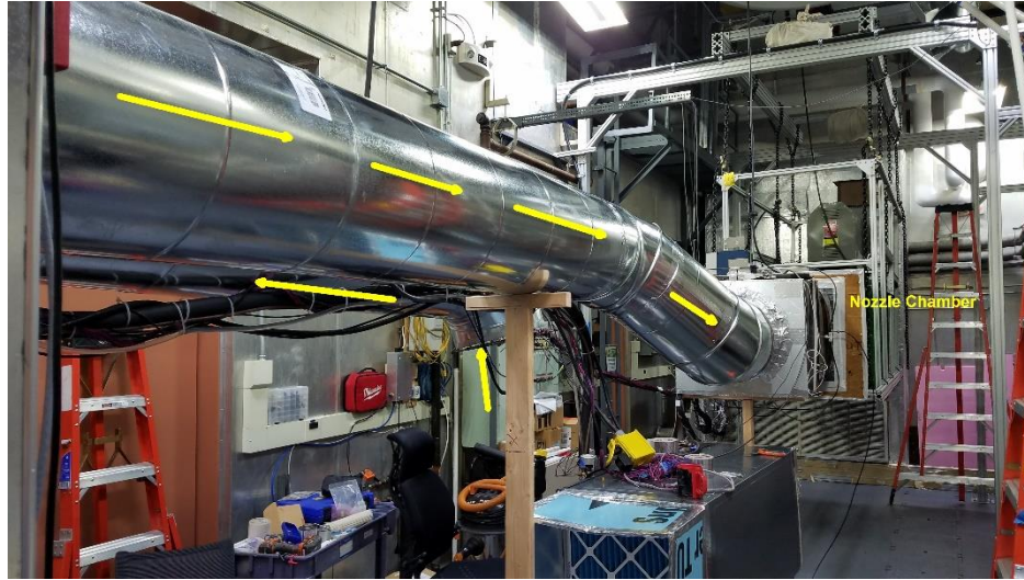
Figure 4.6-4. Connecting ducts and nozzle chamber located in the indoor environmental chamber
