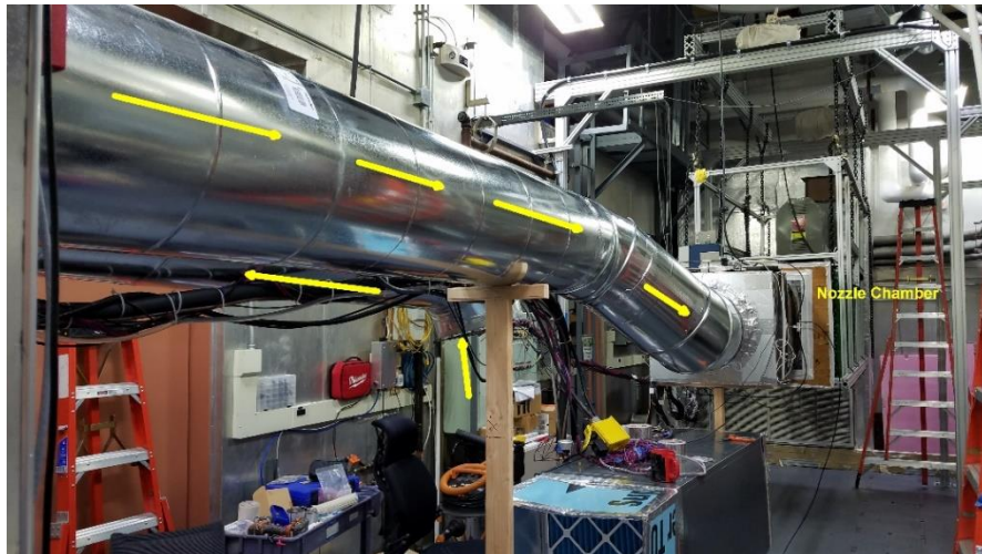
Figure 3 (Exec. Summary). Connecting ducts and nozzle chamber located in the indoor environmental chamber
