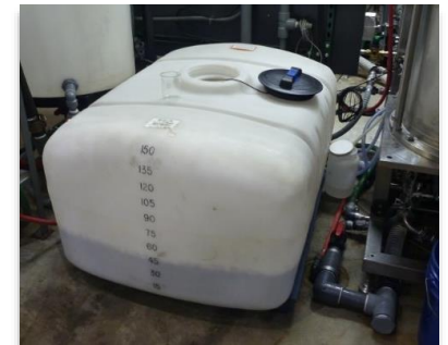
4) Effluent \leq 15 ppm oil sent to drain / wastewater treatment. Effluent > 15 ppm oil sent to underground storage tanks.
