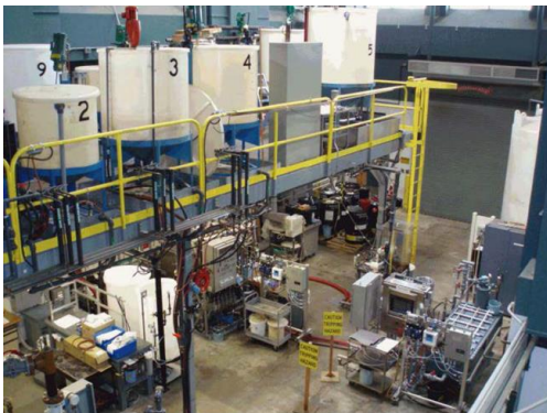
NSWCCD Wastewater Lab
