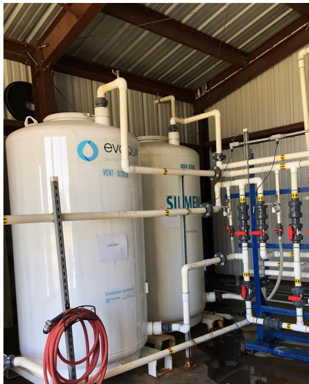
Figure 1: Part of the South pump-and-treat system installed at former Marine Corps Air Base Tustin.
