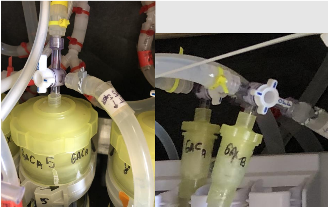
Figure 4: (Left) Top of one of the full-scale columns that is plumbed with a 3-way stopcock to flow either to a passive sampler and then to waste (right tube, marked with gray and white hashed zip tie), or to sample collection (top tube, marked with yellow zip tie). (Right) Top of one of the RSSCT columns plumbed with a 3-way stopcock to flow either to a passive sampler and then to waste (right tube, marked with gray and white hashed zip tie), or to sample collection (left tube, marked with yellow zip tie).
