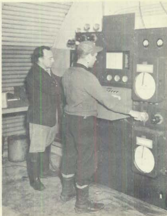
Fig. 3 - Control Panel in Motor Control Room of Test Cell No. 6
