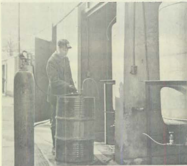
Fig. 4 - 250-gallon Acid and Aniline Fuel Tanks between Blast Walls
