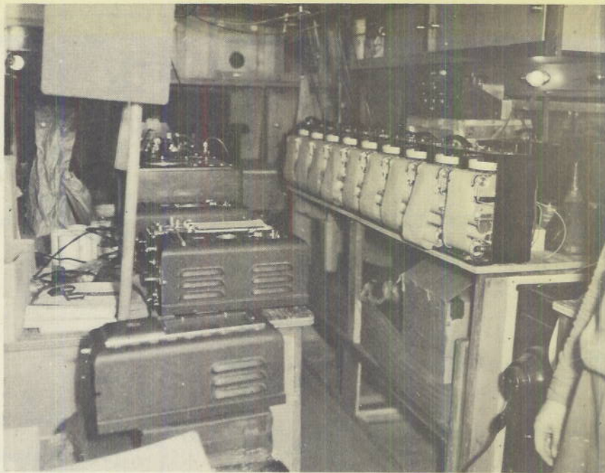
Figure 5 - Interior of Trailer Showing Some of the Receiving and Recording Equipment
