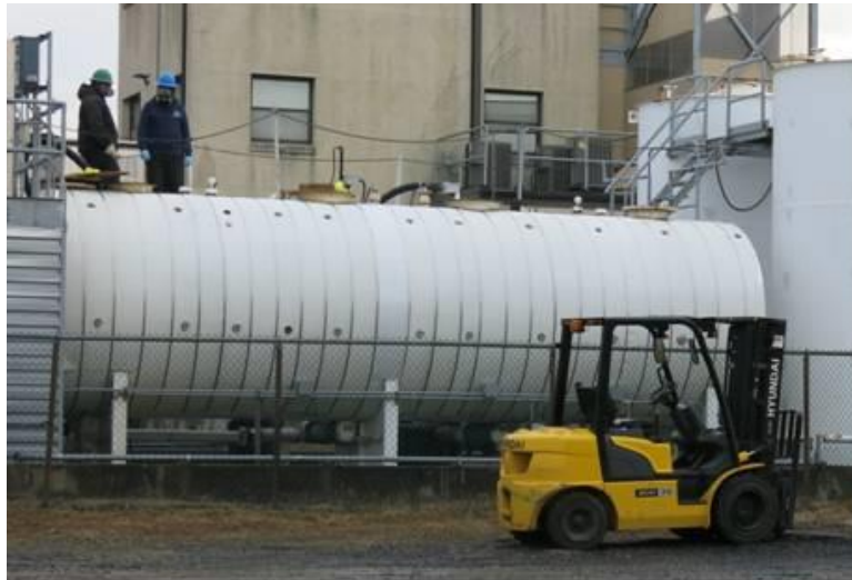
Figure 2. Large tank for large batch of oil (2,000 gallons).
