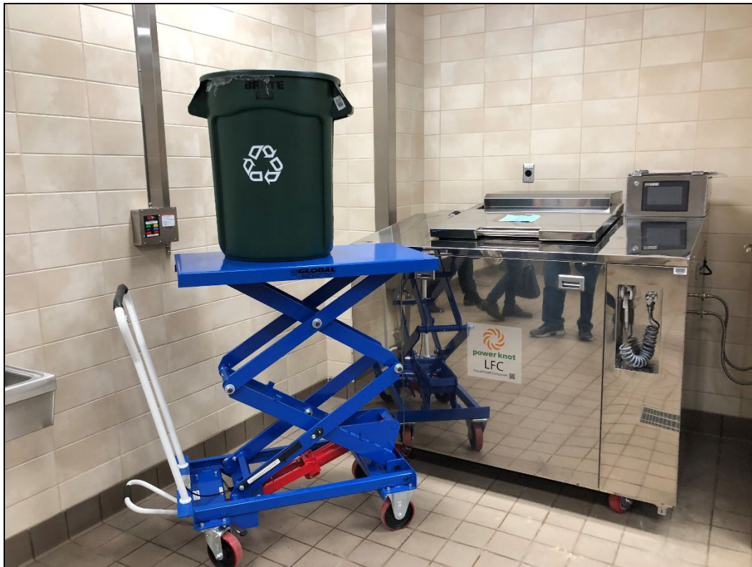
Figure 22. Recycling bin on a lift in front of a liquid digester at Fort Gregg-Adams
