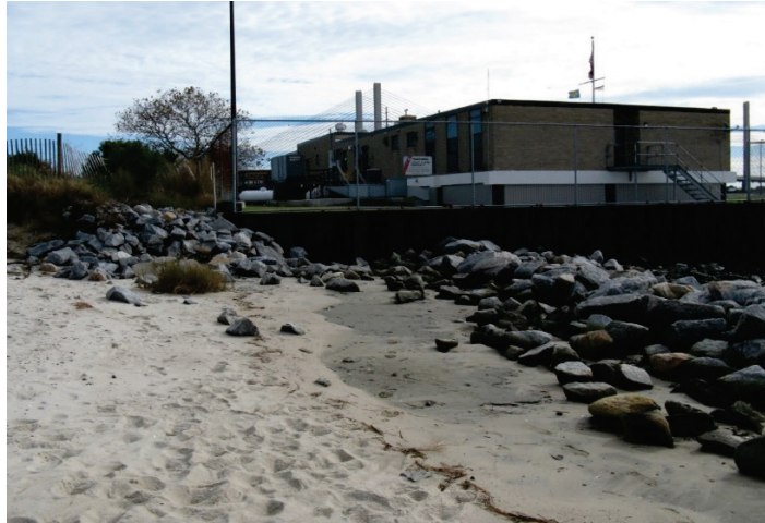
Figure 3. Existing conditions of Bubble gum Beach showing severe escarpment behind the existing riprap (November 2017). (Photo credit: Mark Eberle.)
