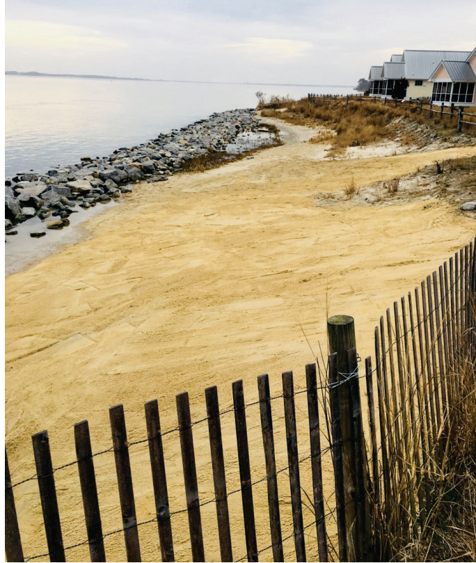
Figure 6. Bubble gum Beach after sand placement was completed in March 2018. (Photo credit: Wayne Marston.)
