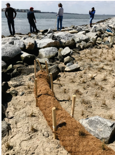
Figure 9. Coir fiber log installed during the April 2018 workshop within the project location. (Photo credit: Danielle McCulloch.)
