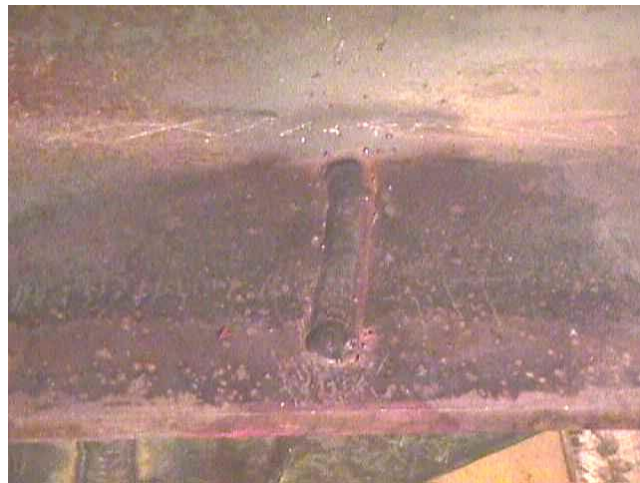
Figure 11-9: Resultant weld between drilled-out crack tips.
