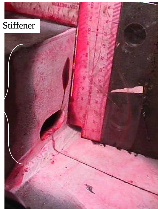
Figure 3-17: Crack growing in stiffener of case 3.
