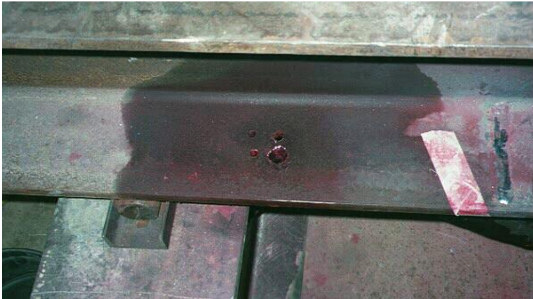
Figure 11-39: Several cracks arrested by hole drilling.
