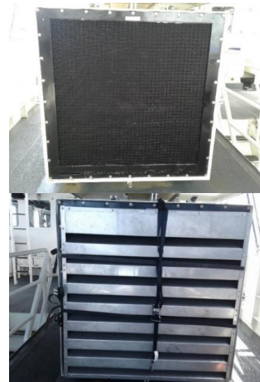
Figure 1. Combustion intake onboard CGC ROLLIN FRITCH without (top) and with (bottom) an acoustical louver (Source: U.S. Coast Guard).
