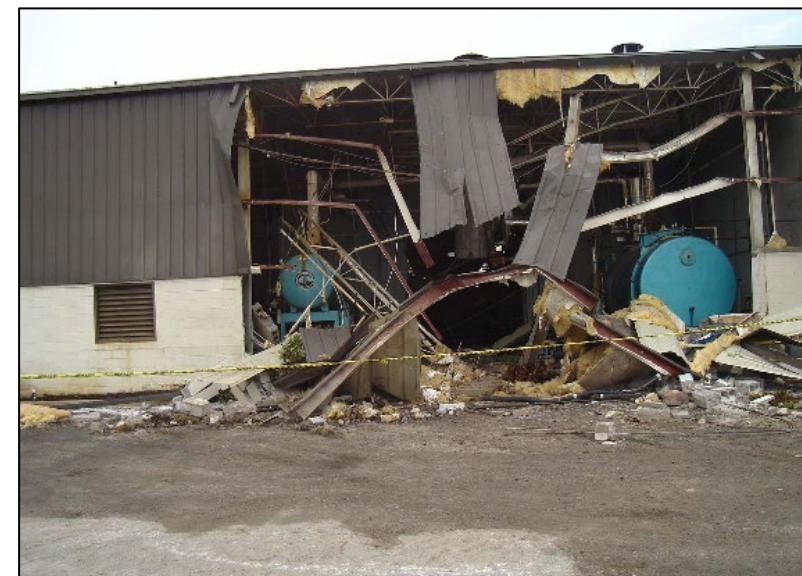
Steam Explosion Dana Corporation plant in Paris, Tennessee
