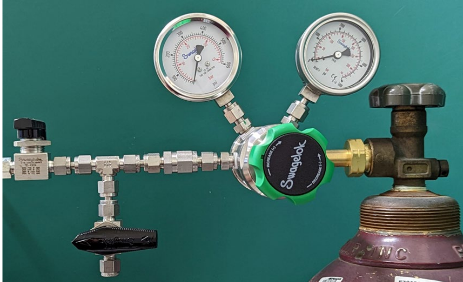
Figure 12. Compressed Air Supply System Control Valves
