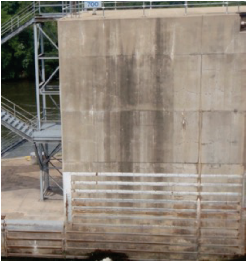
Figure 7. Lockport—Typical restraint cracking in CIP repair concrete.
