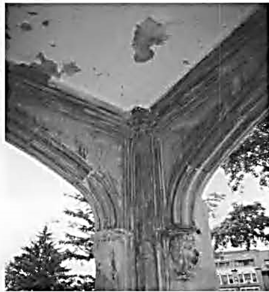
Figure 5. Repeated water washing did not remove the staining inside this limestone porte cochere. Upon closer examination, it was determined to be a water-repellent coating that had been applied many years earlier. An alkaline cleaner may be effective in removing it.
