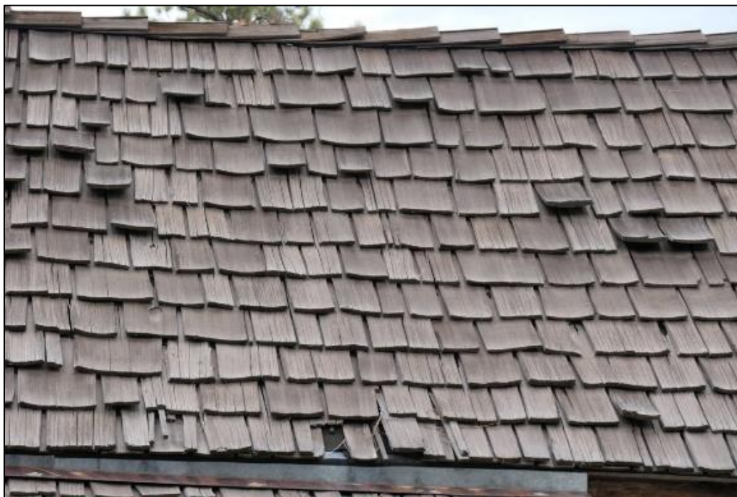
Figure 34. Looking at splitting and curling wood shingles on the south roof side of the Burgess-Capps Cabin (photo by ERDC-CERL researchers, 2021).
