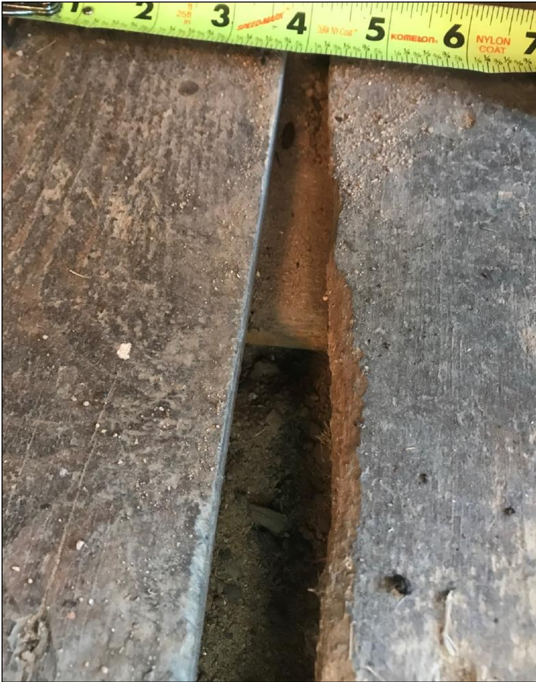
Figure 109. Closeup view showing a floor joist bearing on the soil below (photo by ERDC-CERL researchers, 2021).
