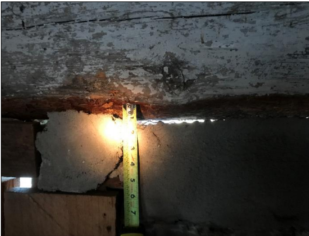
Figure 106. Wall crack (3/4 inch thick) measured just east of the door lintel on the north wall (photo by ERDC-CERL researchers, 2021).
