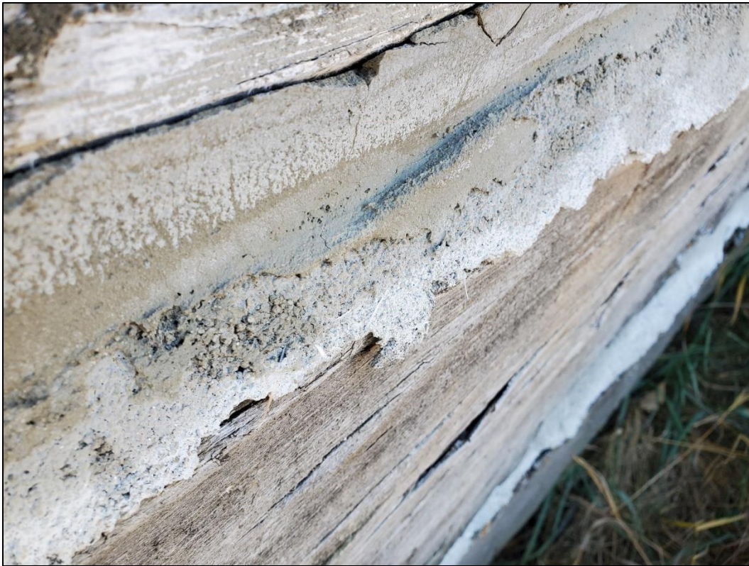
Figure 143. Fiber-reinforced mortar (samples 13 and 18) with white coloration evident of carbonation (photo by ERDC-CERL researchers, 2021).
