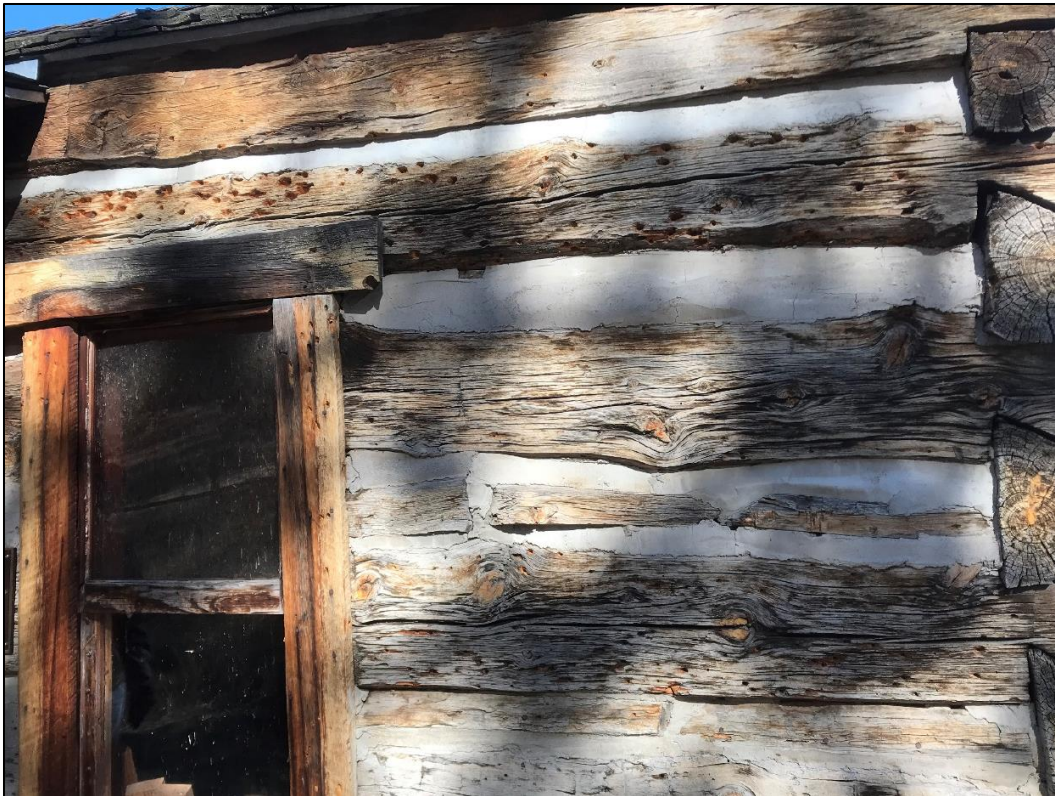
Figure 102. East side of the south wall showing the timber and mortar condition (photo by ERDC-CERL researchers, 2021).
