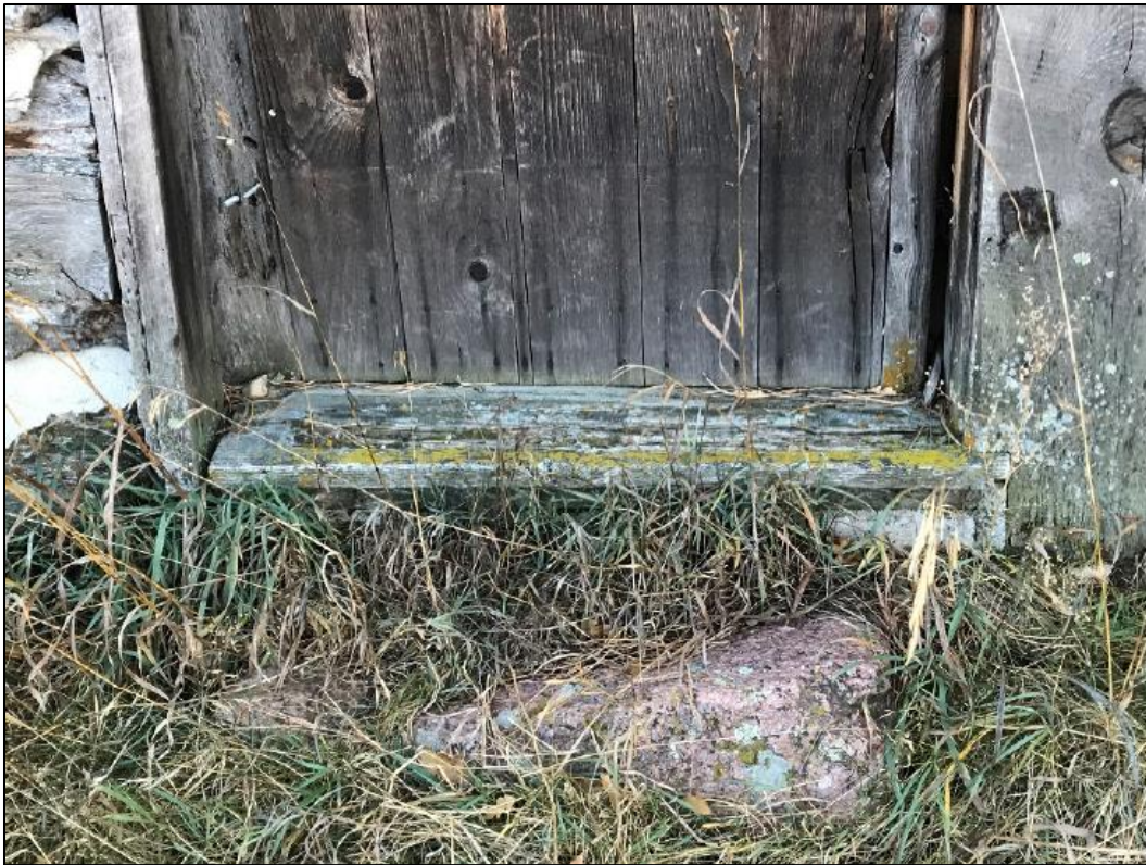
Figure 107. Rotted north door framing, including the threshold (photo by ERDC-CERL researchers, 2021).
