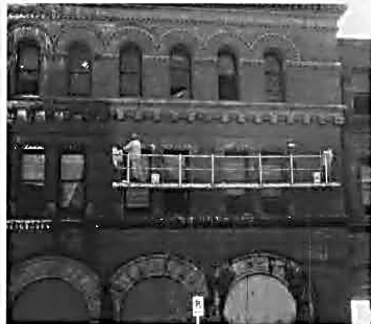
Figure 12. A mild acidic cleaning agent is being used to clean this heavily soiled brick and granite building. Additional applications of the cleaner and hand-scrubbing, and even poulticing, may be necessary to remove the dark stains on the granite arches below. Photo: Sharon C. Park, FAIA.
