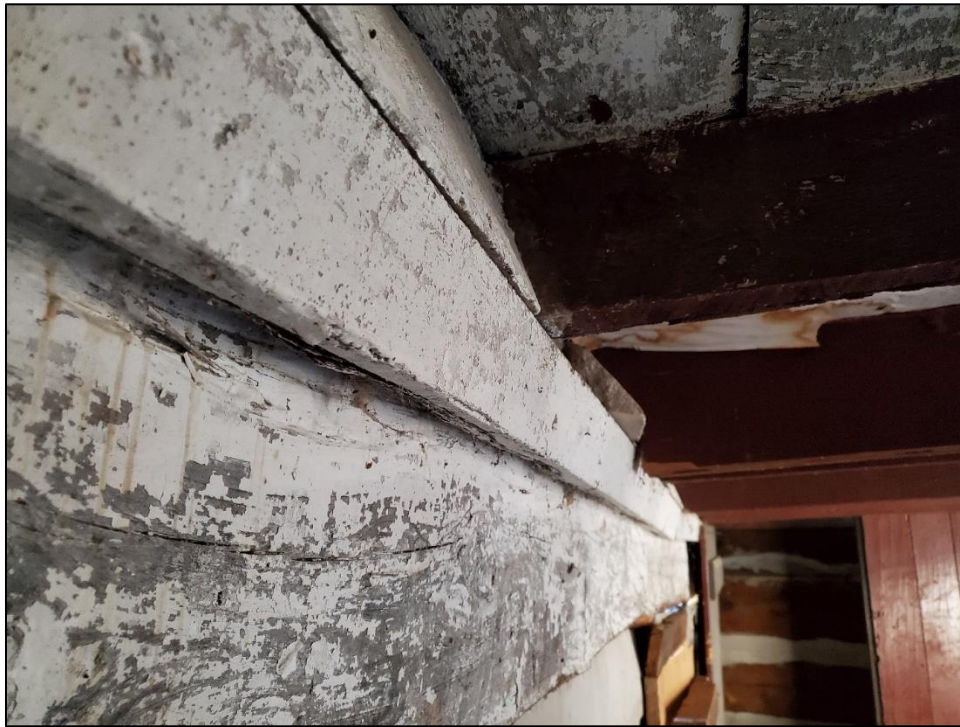
Figure 150. A combination of a rough-sawn or hewn, true-dimensional joist and a notched, sistered dimensional lumber joist (photo by ERDC-CERL researchers, 2021).
