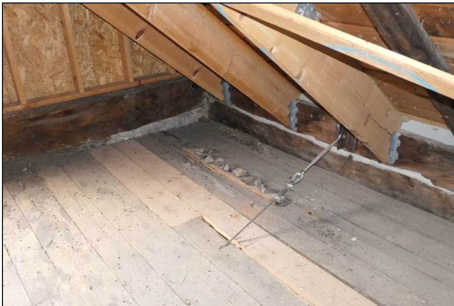
Figure 90. Turn-buckle and cable that is fastened to a double 2 × 8 below the loft floor, which connects to a turnbuckle, which is bolted to two steel angle brackets, which are lag bolted to the top wall timber in the loft of the Burgess-Capps Cabin (photo by ERDC-CERL researchers, 2021).
