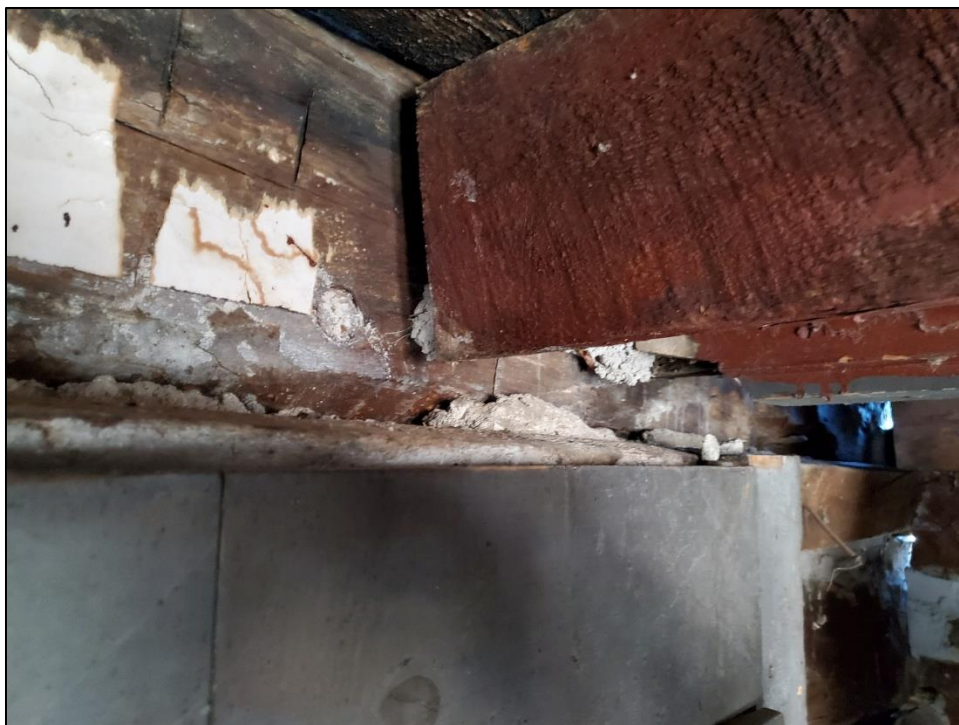
Figure 151. Example of a poor connection between the north wall plate and the ceiling joists (photo by ERDC-CERL researchers, 2021).
