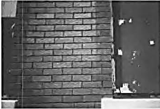
Figure 18. The glazed bricks in the center of the pier were covered by a signboard that protected them being damaged by the sandblasting which removed the glaze from the surrounding bricks.
