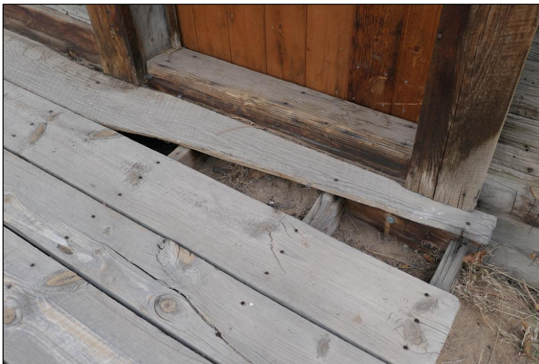
Figure 49. Split and broken wood planks and wood joists that make up the porch floor of the Burgess-Capps Cabin (photo by ERDC-CERL researchers, 2021).
