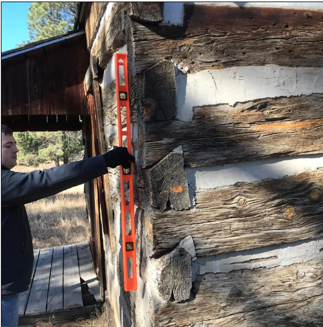
Figure 103. Southeast corner of the cabin showing the south wall leaning outward away from the building (photo by ERDC-CERL researchers, 2021).
