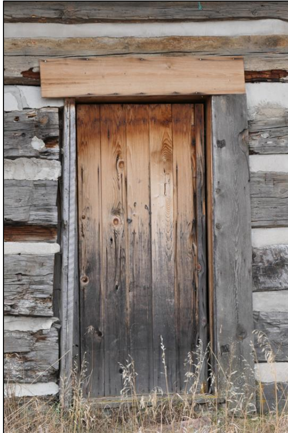
Figure 41. Looking at a combination of old and new wood door trim of different sizes on the north elevation of the Burgess-Capps Cabin. There is also a missing plank on the left side of the door (photo by ERDC-CERL researchers, 2021).
