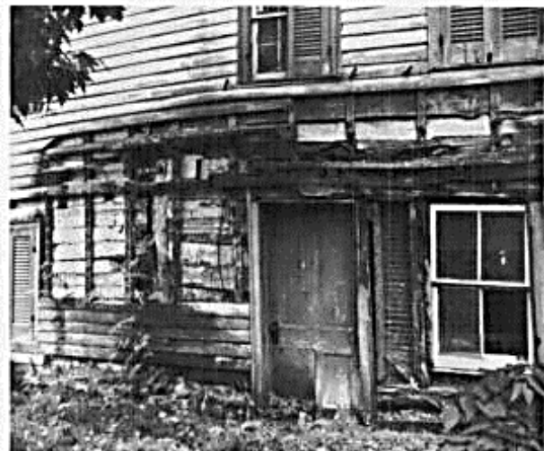
Fig. 17. Contact of this building's sill log with the ground has led to its decay, infestation by wood-destroying insects, and resulting building settlement. Photo: Anne Grimmer.
