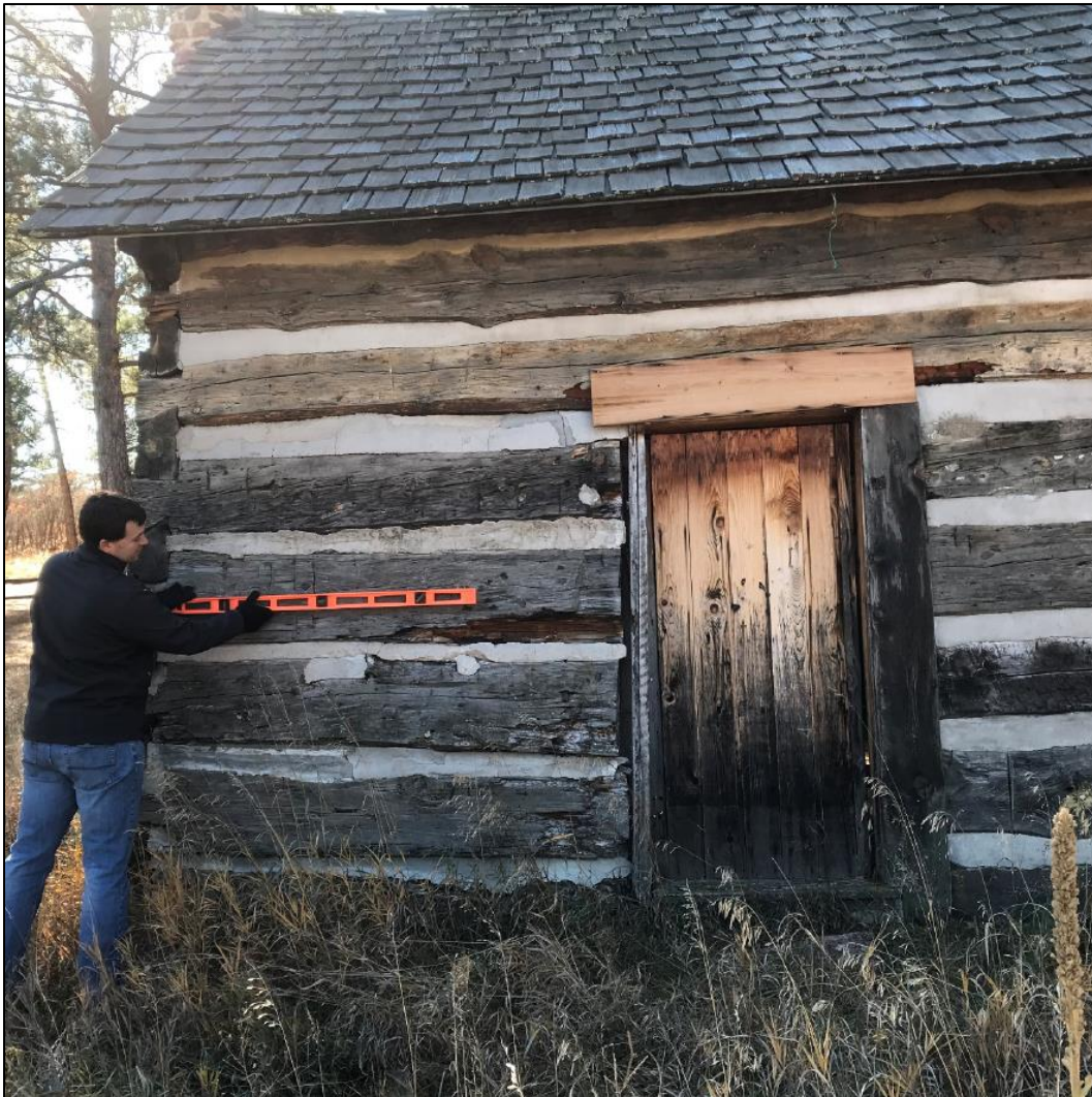
Figure 105. East portion of the north wall where considerable timber rot and settlement was seen (photo by ERDC-CERL researchers, 2021).
