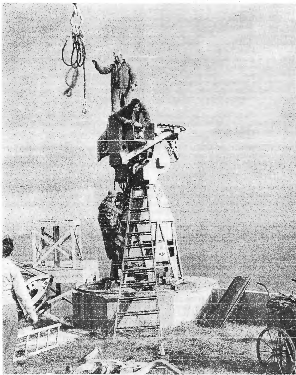
"On location" at the Chesapeake Bay Annex, NRL's field test station, Randle Cliff, Md. Here a skilled construction crew, supervised by Laboratory technologists, erects an experimental radar antenna for trials over the seascape.
