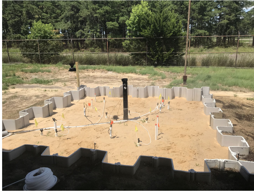
Figure ES1. Installed 14 ft x 14 ft test cell.
