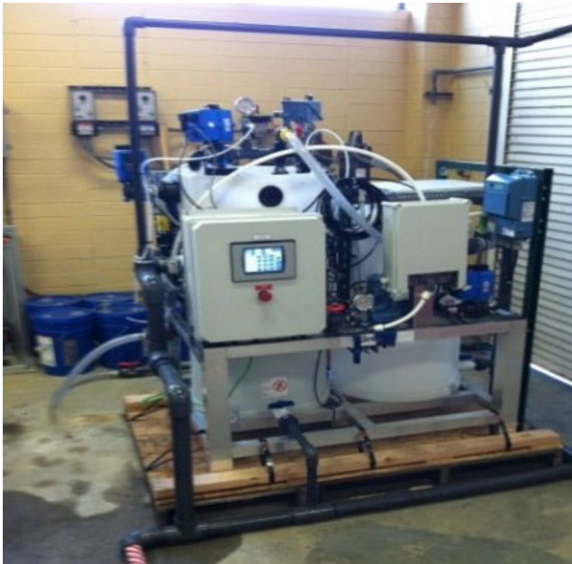
Figure 3.1 Photo of Electrochemical Disinfection pilot system under NESDI 487.
