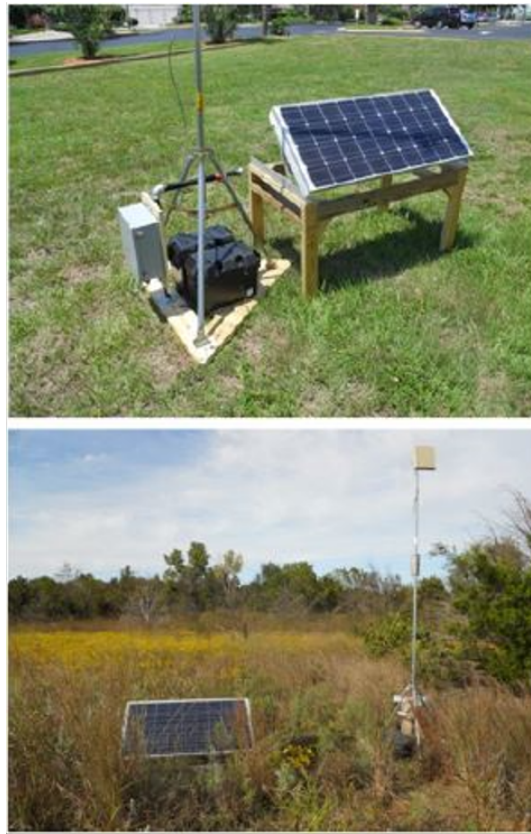
Figure 25. A View of the Node and Battery Assembly with the Solar Panel (Top), and an Installed at Ft. Sill (Bottom).
