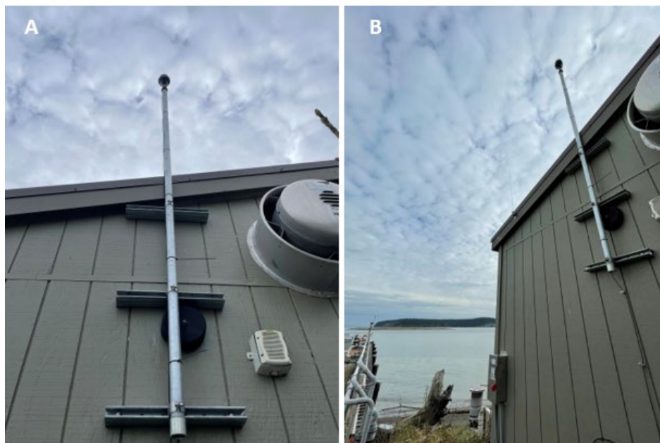
Figure 10. RTK GNSS receiver mounted on the building on PNNL-Sequim's campus.
