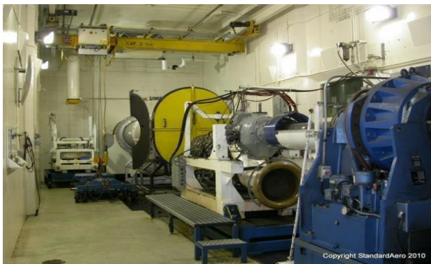
Figure 10: Engine Test Facility at SA WPG
