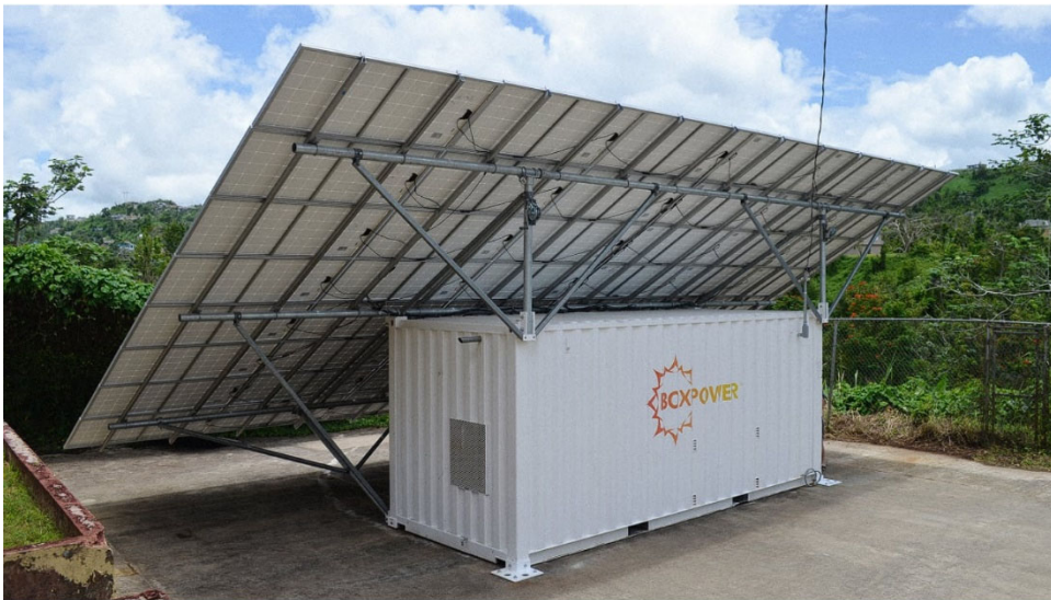
Figure 42 The Boxpower solar container microgrid [65].
