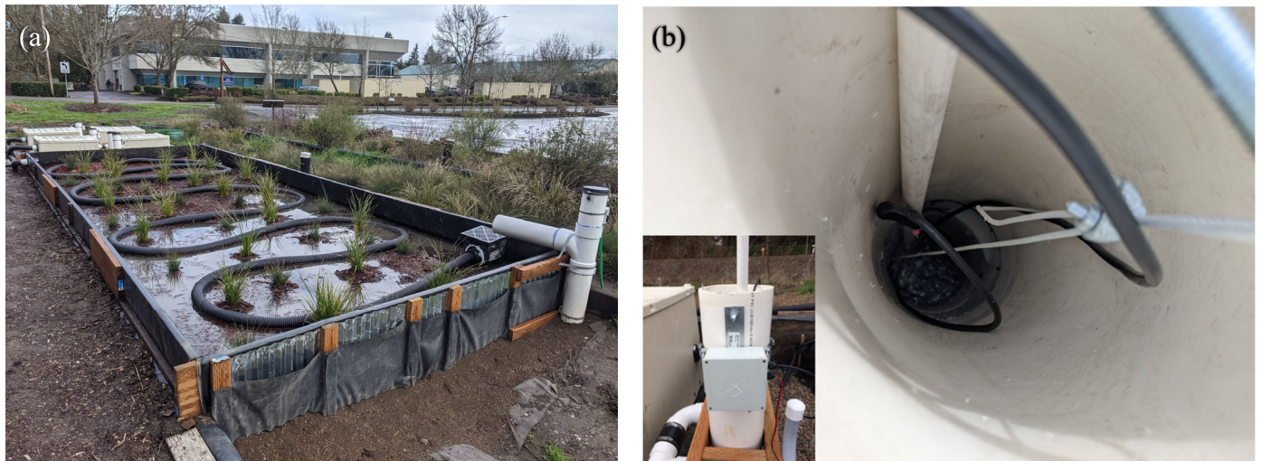
Figure 8: (a) Completed treatment train; (b) Installation of Flow and Turbidity in-situ sensors in risers for real-time monitoring to support Task 3.2, 4.1 and 4.2.
