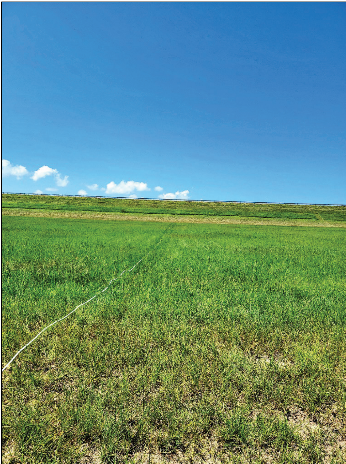
Figure 11. DAA-3 ( foreground , levee flat) and DAA-4 ( background , levee slope) that were assessed as USACE infrastructure where feral swine damage had been identified by local staff at the Somerville Lake project, Texas.
