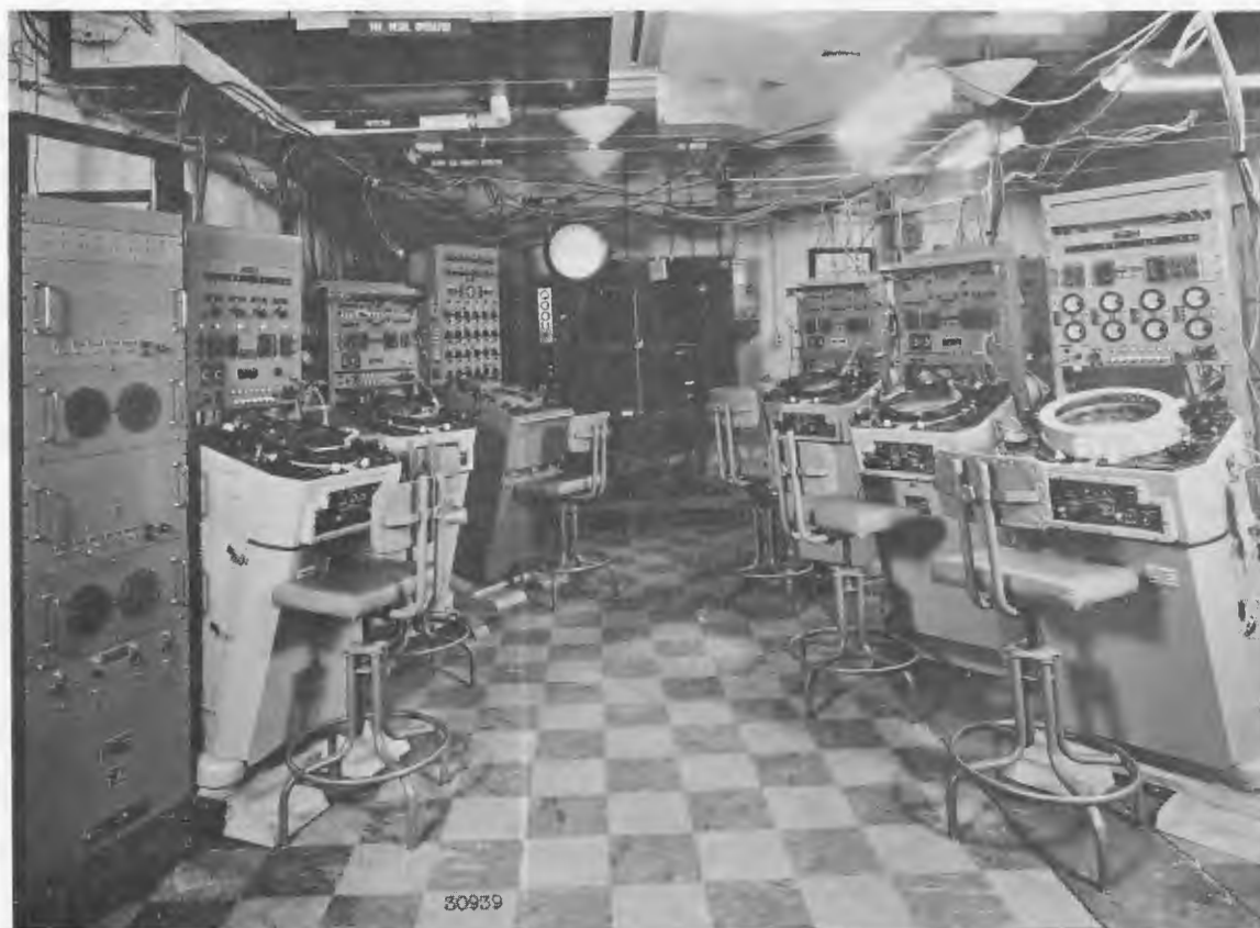
Fig. 17 - The Electronic Data System installation at the Chesapeake Bay Annex. From left to right are the Target Designation Rack and Console, the Supervisor (detector) console, the HSI console, the ASPB, Tracker No. 1 console, Tracker No. 2 console, and the Air Intercept Controller console.
