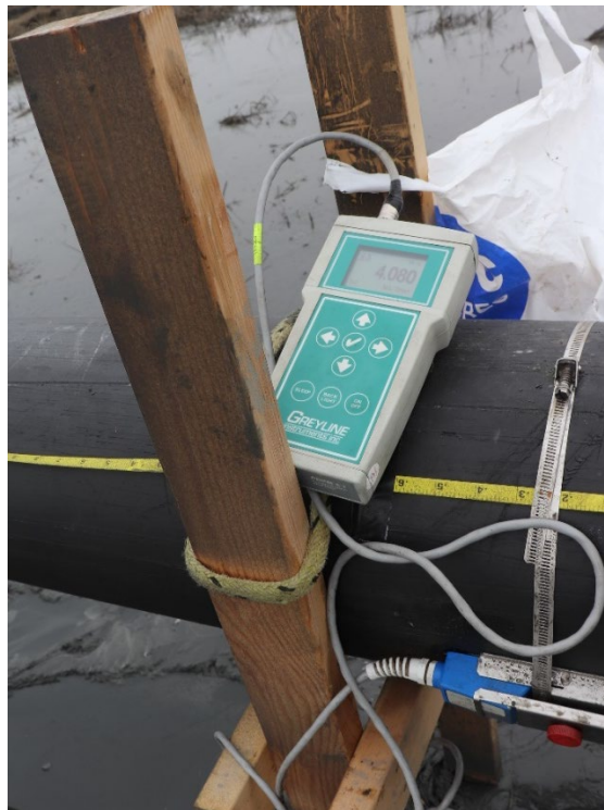
Figure 8. Greyline 5.1 noncontacting Portable Doppler Flow Meter (PDFM) with ultrasonic sensor clamped to pipeline.
