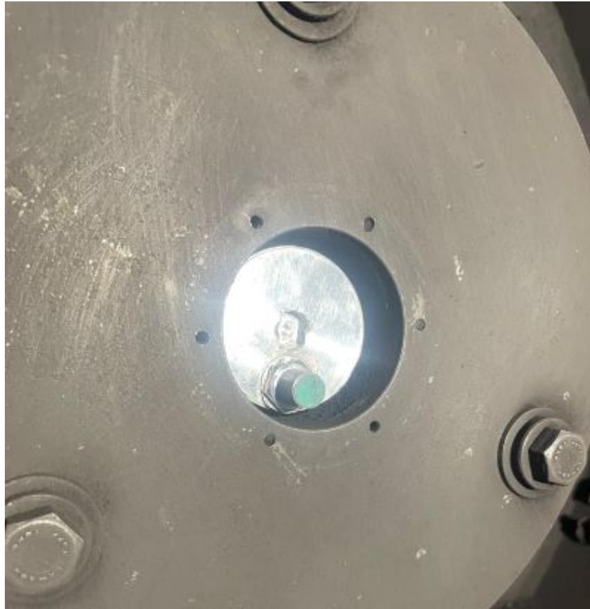
Figure 3.20. Proximity Sensor Check
