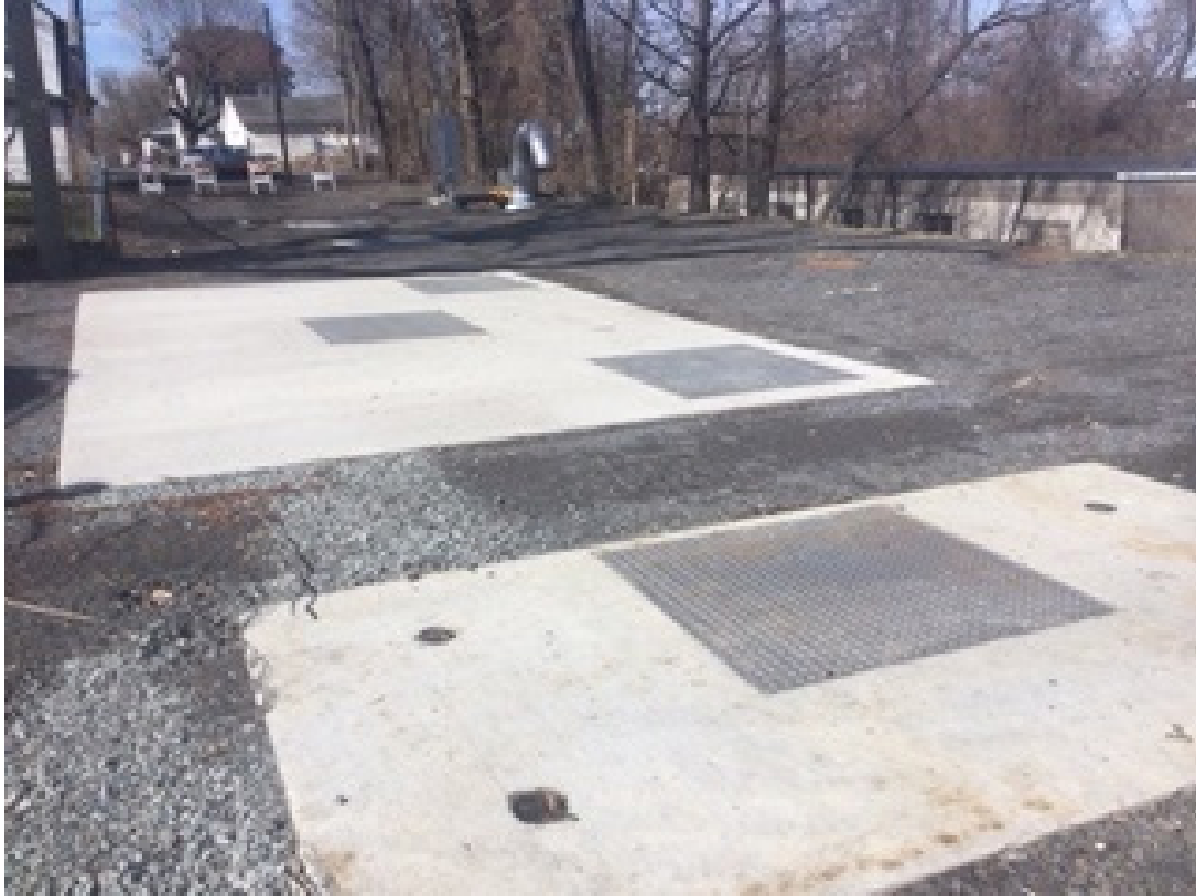
Figure 12. Scranton Stormwater Street Vaults 306
