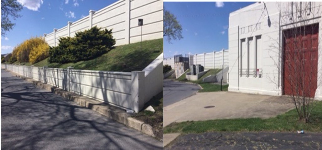
Figure 10. Wyoming Valley Levee System 301
