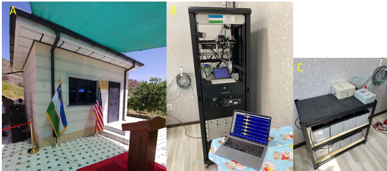
Figure 16. A) Recording room building from outside. B) Equipment rack (and laptop showing seismogram). C) Battery backup.
