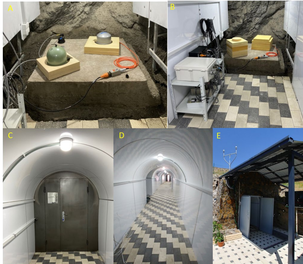
Figure 15. A). Seismic pier with seismic sensors (uncovered for clarity). B) View of seismic vault showing sensors and digitizers (at left). C) Outside of vault door. D) Looking down tunnel towards entrance (from inspection trip). E) Outside of tunnel. GPS antenna at top.
