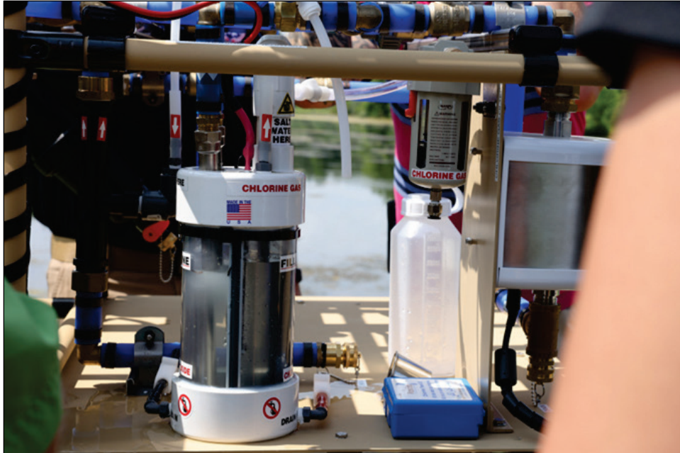
Figure 4. The DRIPS unit's integrated electrochlorinator from WaterStep. The M100 supplies the gas infusion of chlorination into the water treatment train, providing rapid disinfection to the source-water treatment.
