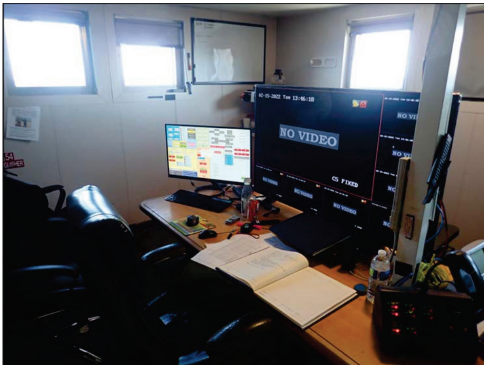
(a) Main operational control room
