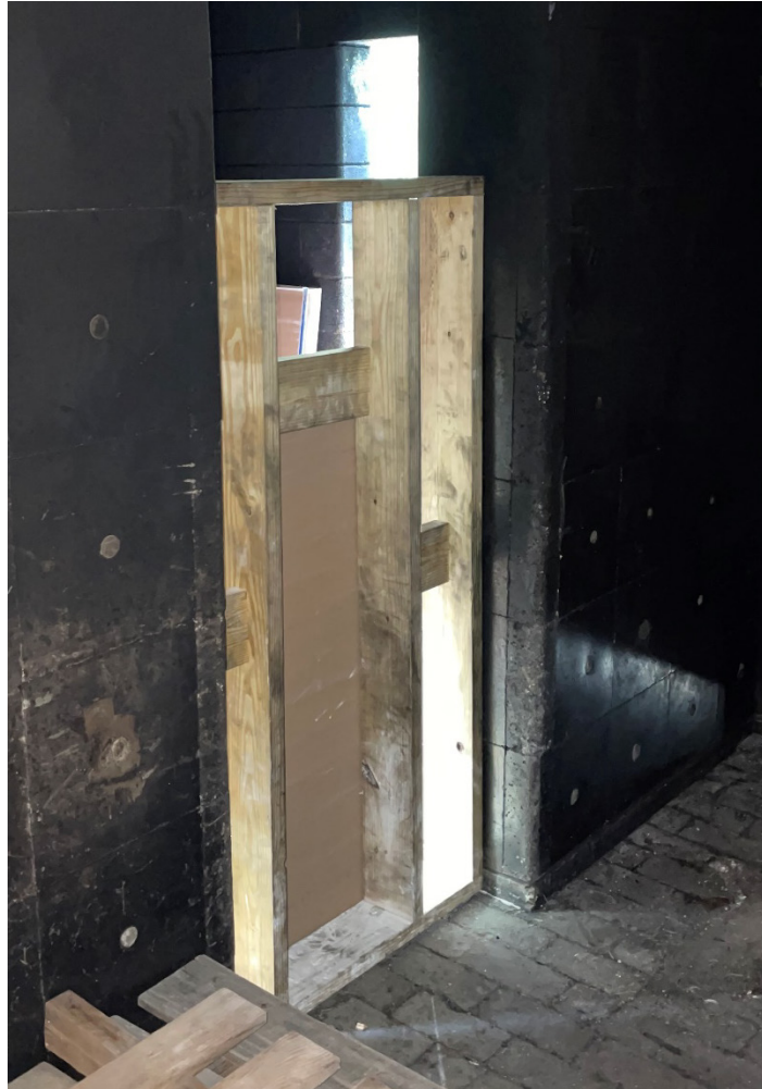
Figure 12. Wall breach prop
