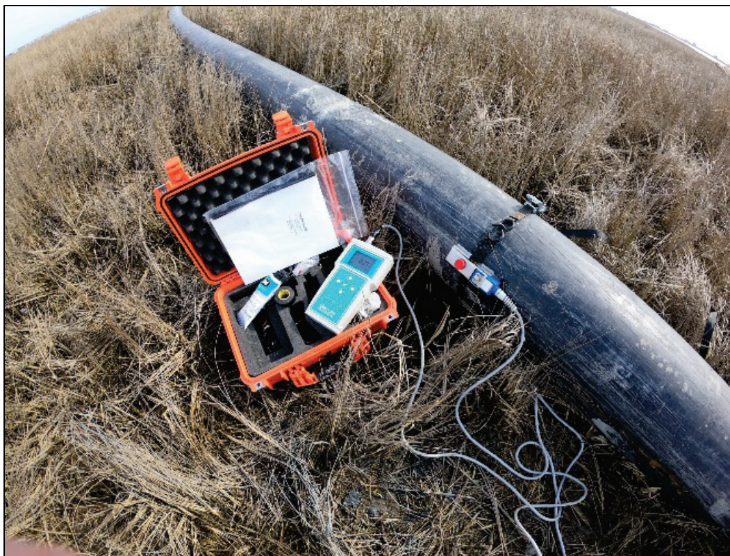
Figure 12. Greyline 5.1 noncontacting portable doppler flow meters (PDFM) with ultrasonic sensor clamped to pipeline.
