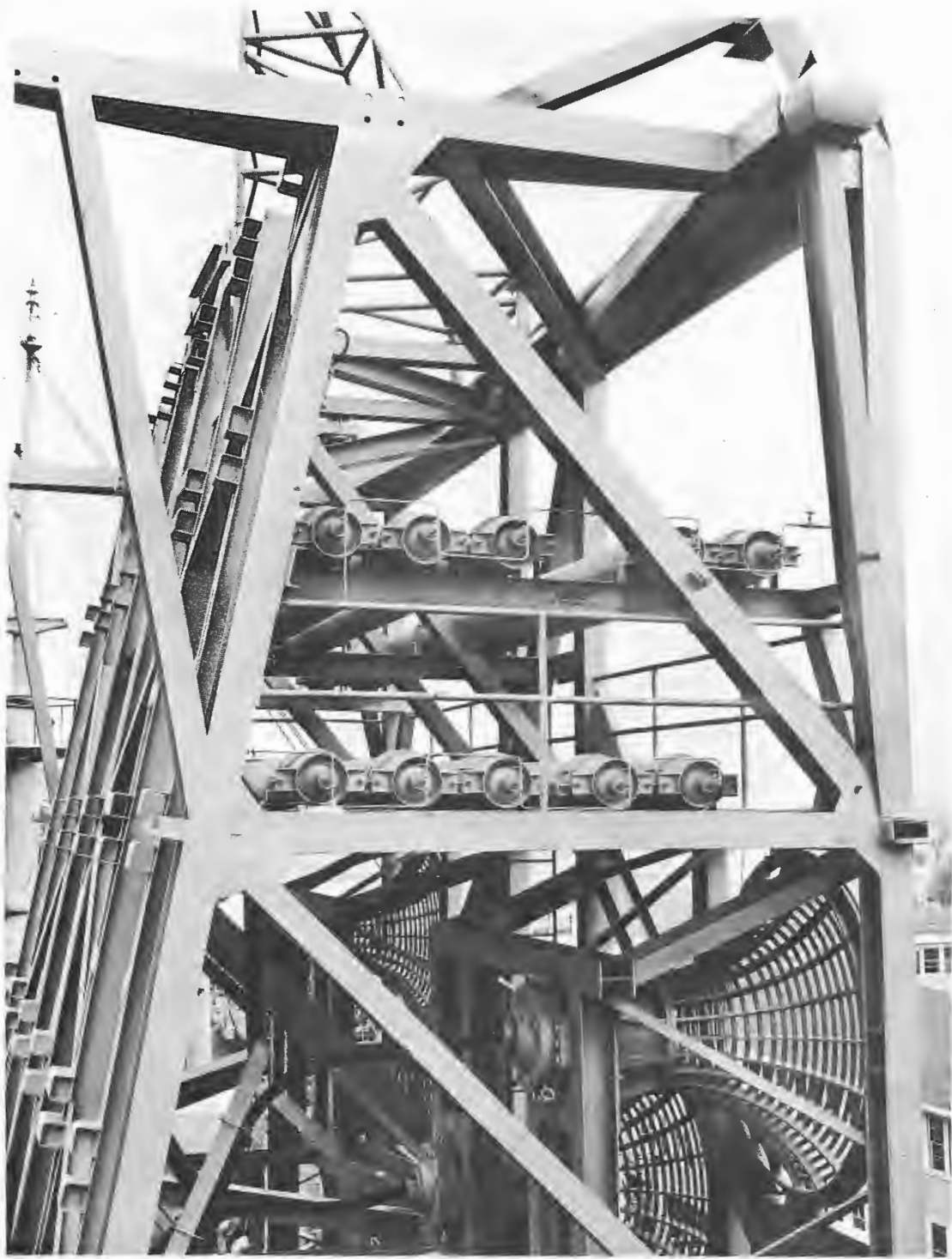
Figure 70 - Array structure viewed from forward showing nitrogen bottles and electric cable entrance bells
