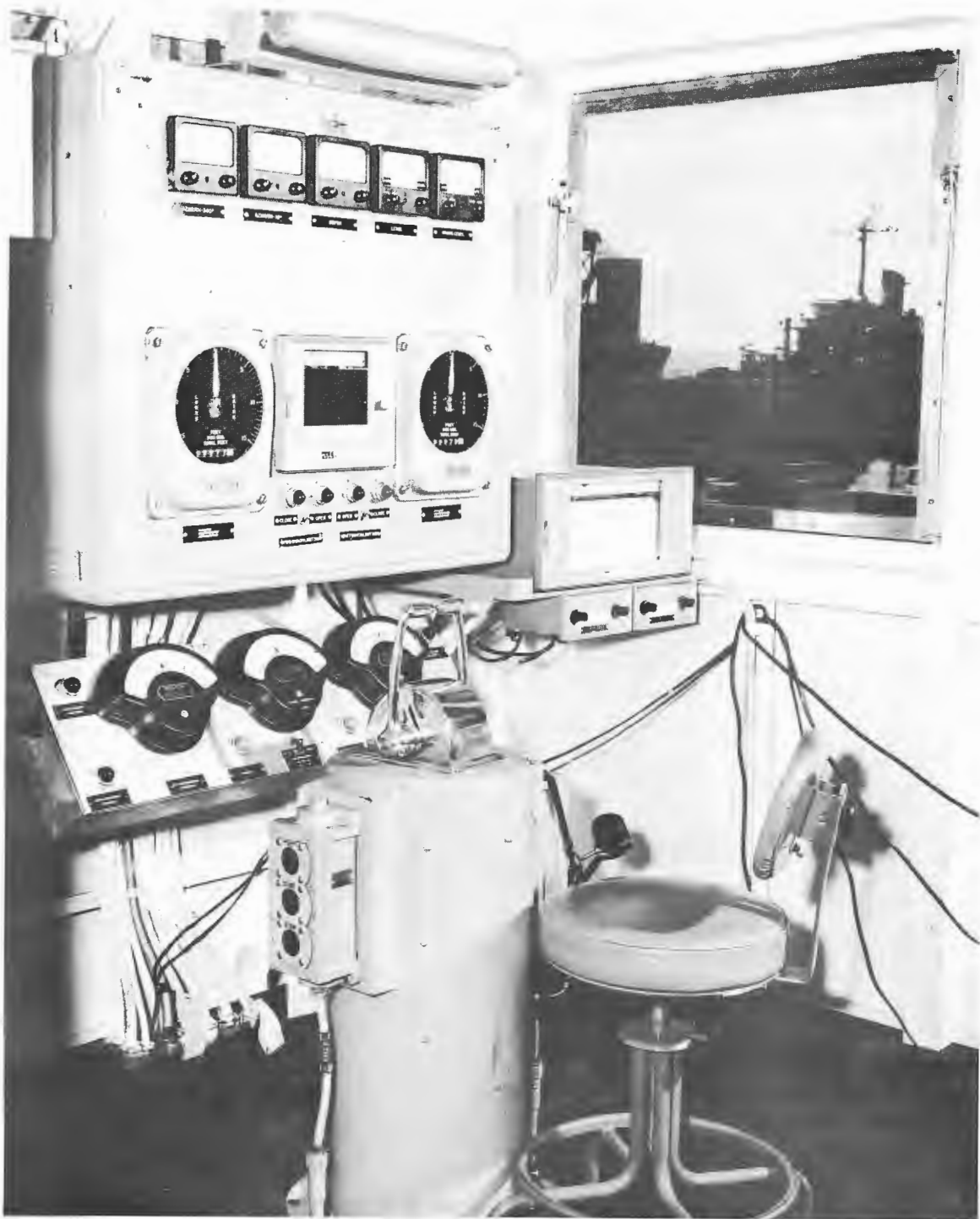
Figure 59 - Array control station off of midship deck house at 02 level; controls for fore and aft array winches
