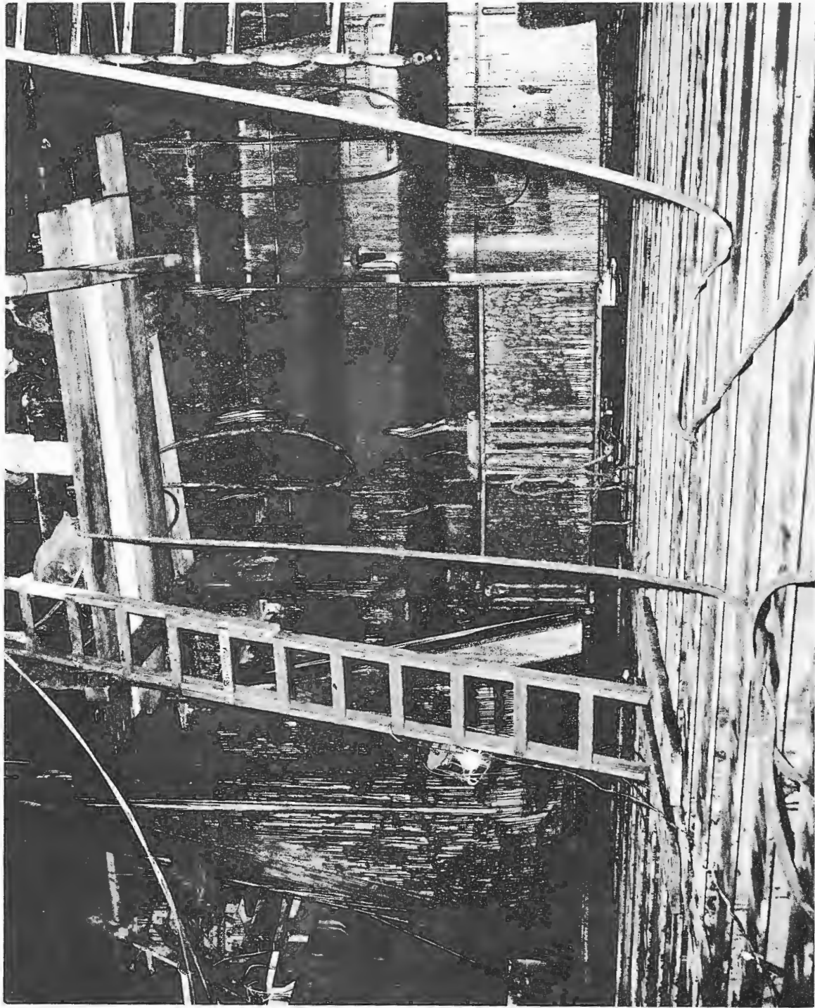
Figure 37 - Array shock mounted guide and cable roller path guide support looking forward
