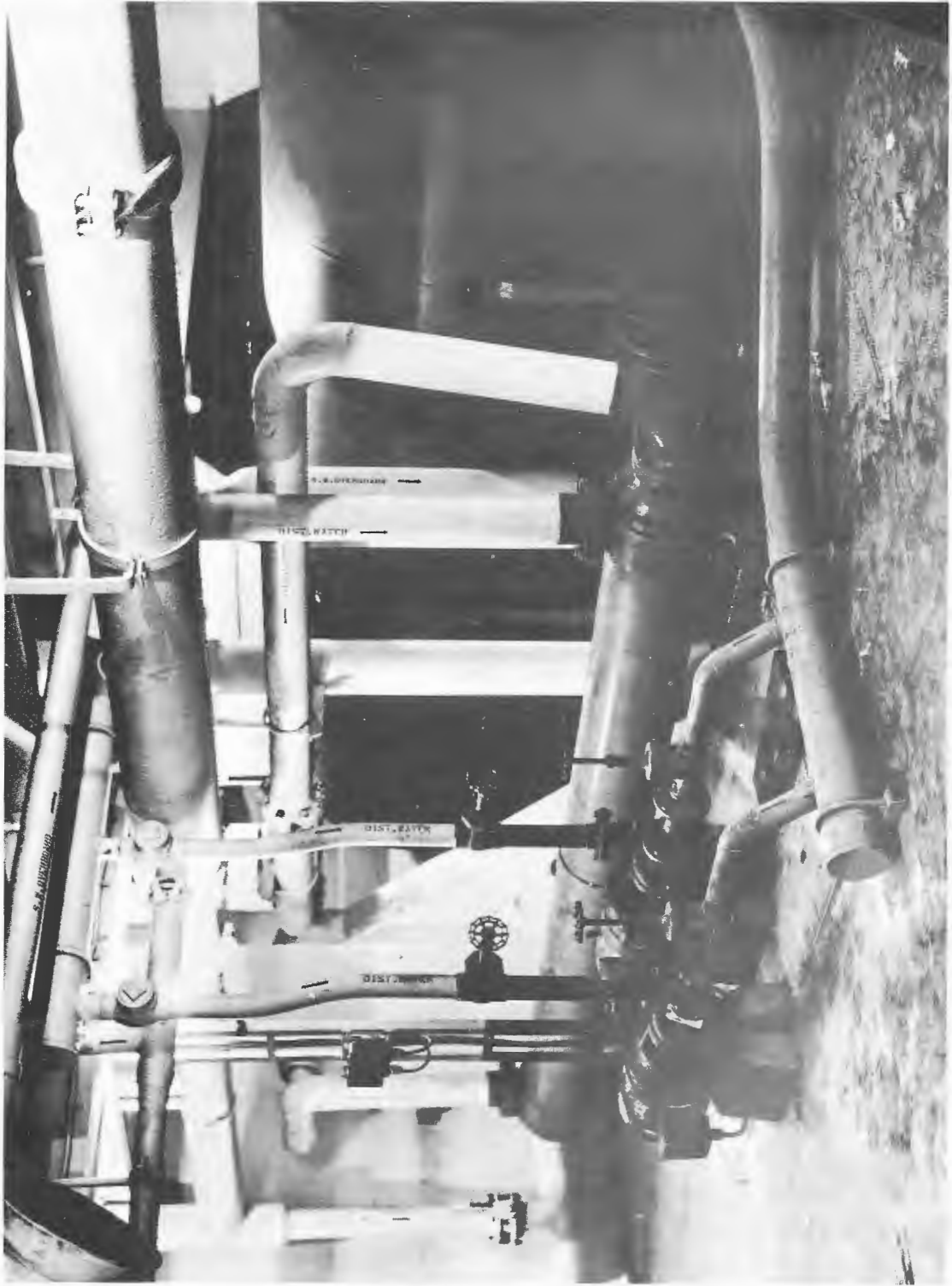
Figure 50 - Single amplifier and system test load cooling water
