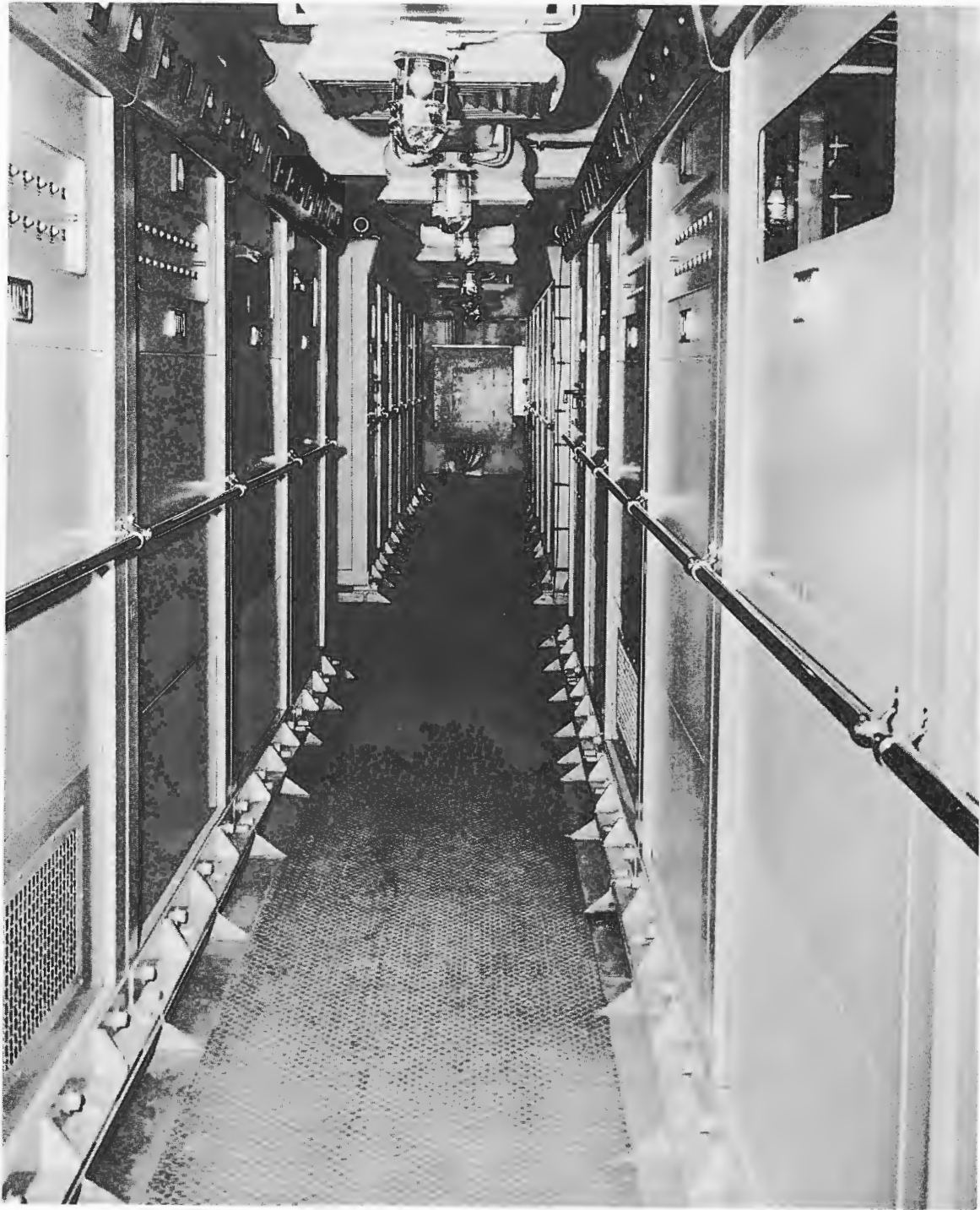
Figure 46 - Front view of four Ling amplifiers
