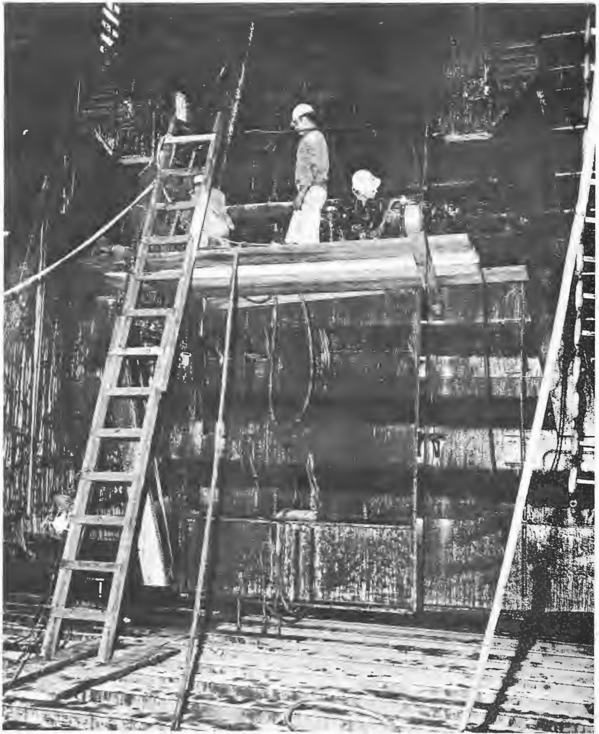
Figure 38 - Array shock mounted guide and cable roller path guide support looking forward
